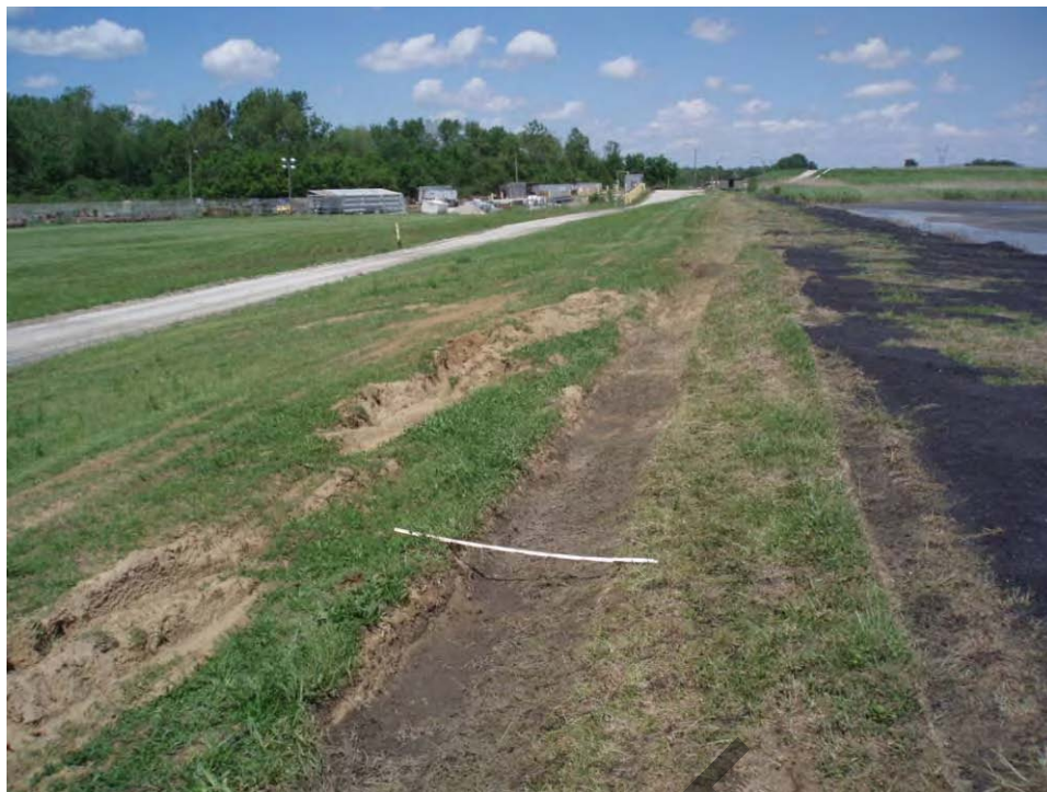
27. Pond A - West embankment exterior slope, looking north at large tractor ruts and excavator tracks.
