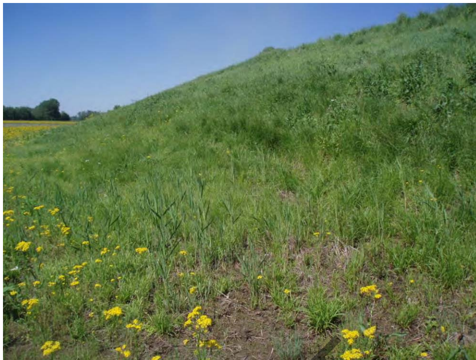
73. Pond B - West embankment lower exterior slope, looking north at saturated area at toe of slope.
