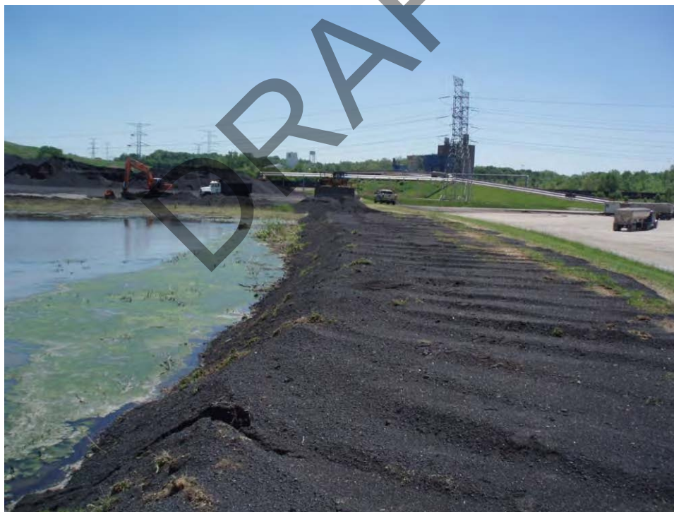
16. Pond A - South embankment crest, looking southeast at recently placed ash material. Note existing embankment was not cleared or grubbed before placing material.
