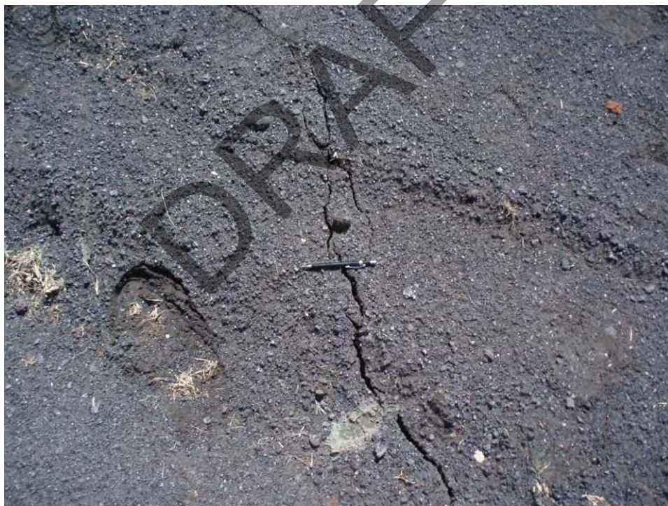
18. Pond A - Surface cracks in recently placed ash material on south embankment crest.
