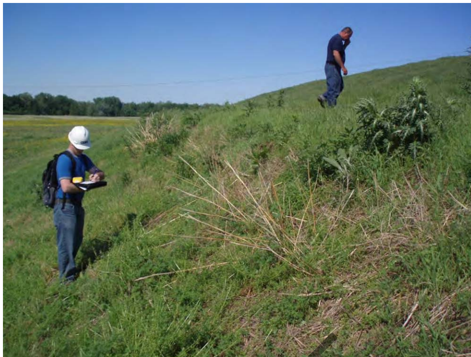
87. Pond B - West embankment lower exterior slope, looking north at over-steep slope and tractor ruts near bench.
