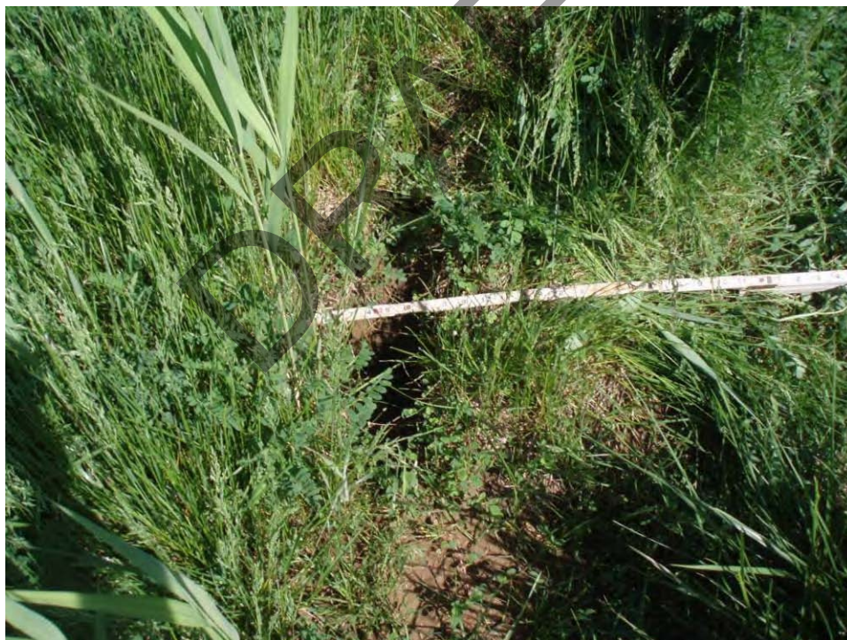
86. Pond B - West embankment upper exterior slope, looking at an 8-inch-diameter rodent hole.
