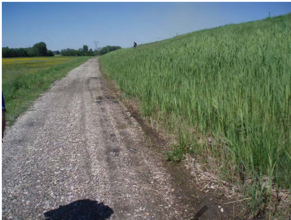
79. Pond B - West embankment bench, looking north at possible seep. Note area is soft and saturated.
