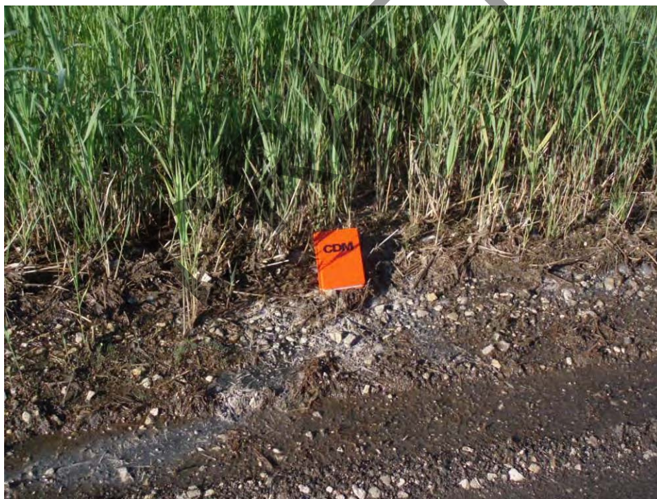
122. Pond C - North embankment bench, looking at active seepage located at toe of upper exterior slope. Note the white sheen in the water.
