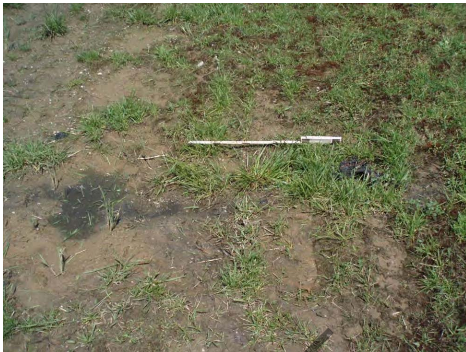
25. Pond A - Saturated area on west embankment exterior slope.
