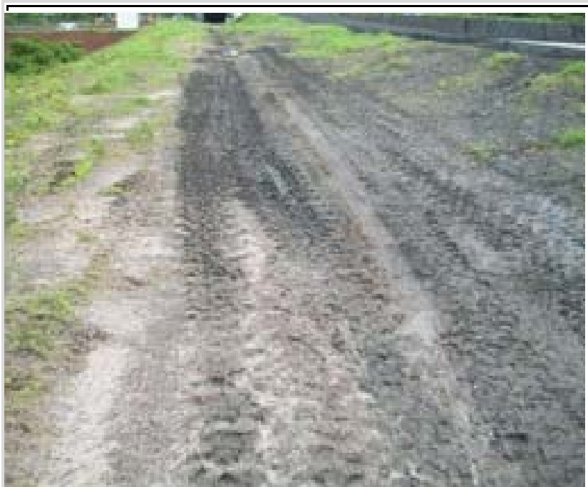
Fig. 5.2.1-1. Water ponding on west embankment buttress
