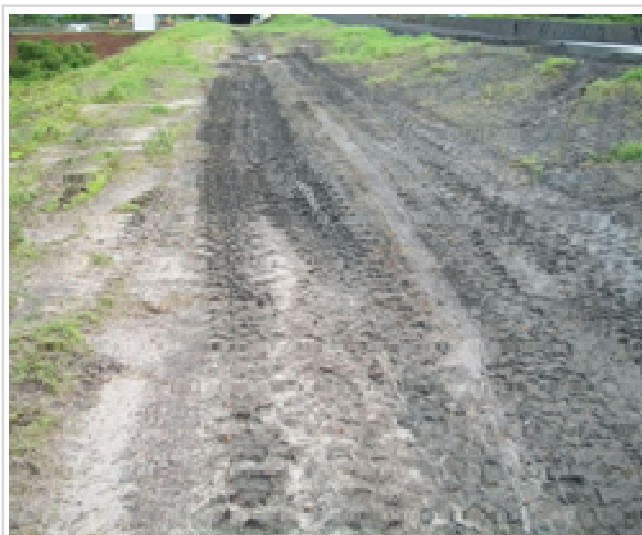
Photo 6 West embankment buttress fill (Old road bed) ponding water
