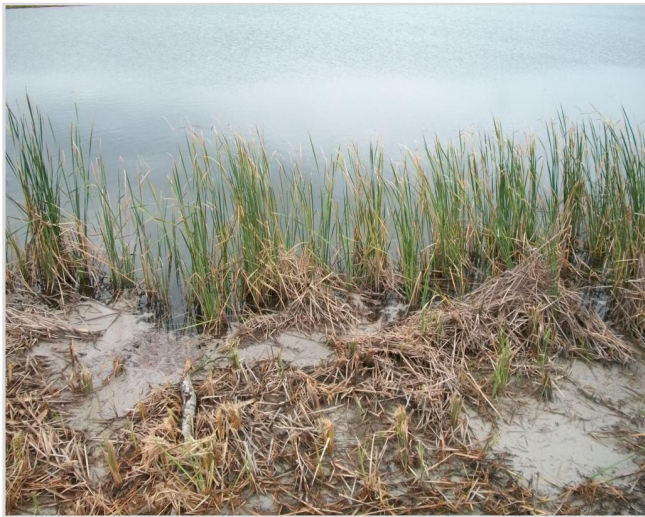
Photo 26 Cattails recently trimmed on East embankment interior
