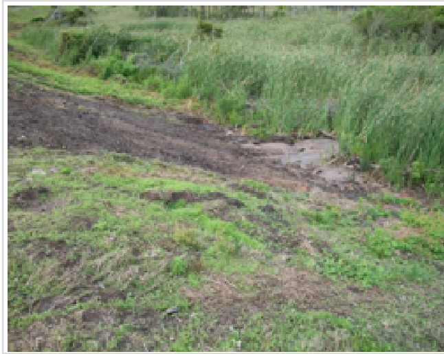
Photo 8 Recently fixed Sloughing on West embankment
