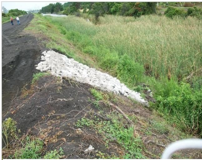
Photo 28 Rip rap repair of North embankment near North East corner and adjacent to recycle canal
