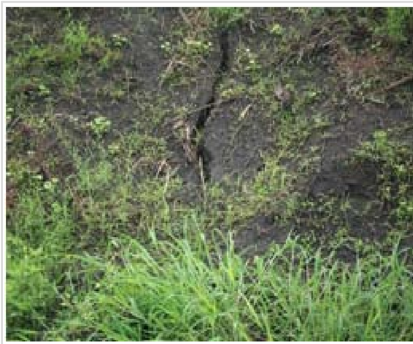
Fig. 5.2.3-1. Rill erosion along downstream slope of west embankment.
