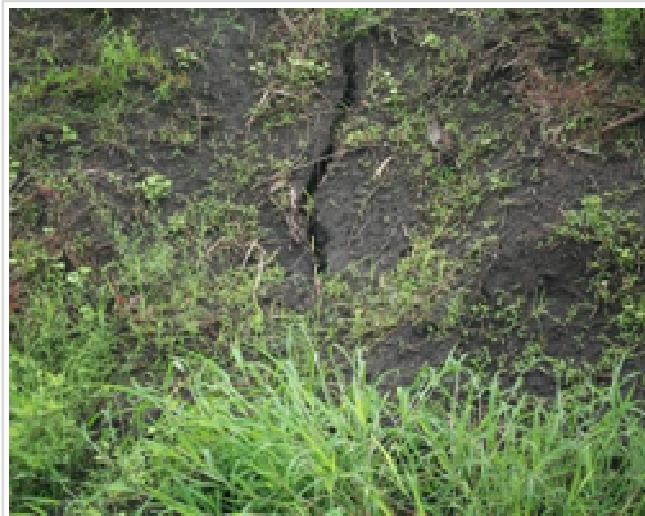
Photo 7 Rilling on slope of West embankment
