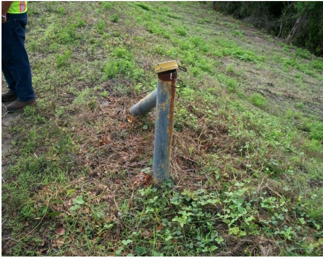
Photo 17 Abandoned test well at top of banks on South embankment
