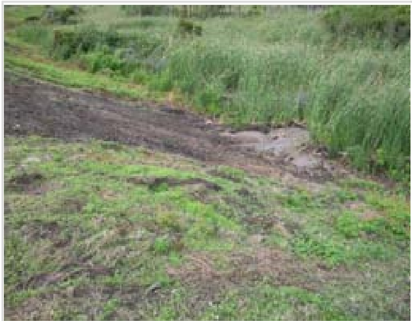
Fig. 5.2.3-2. Recently fixed sloughing on west embankment.
