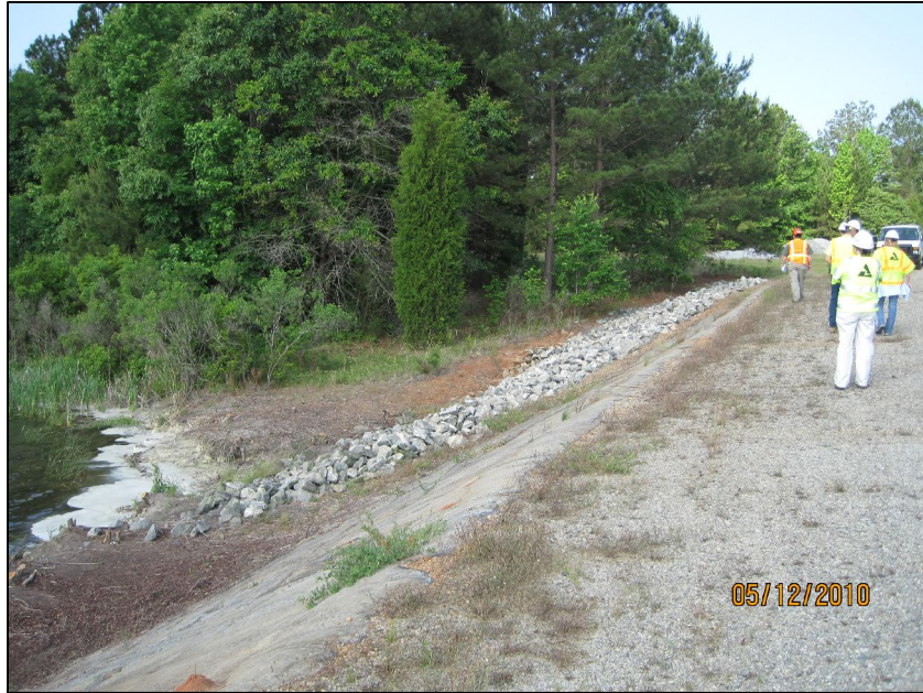
AP-11 CREST OF NORTH DIKE, LOOKING AT UPSTREAM SLOPE AT LEFT ABUTMENT TIE-IN
