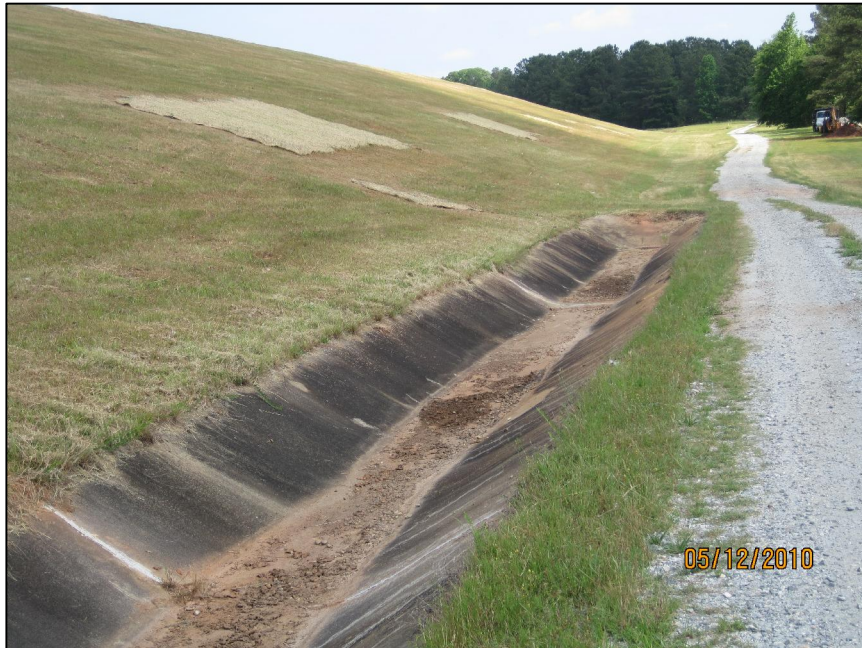
AP-24 LOWER DOWNSTREAM SLOPE OF EAST DIKE, LOOKING NORTH, END OF CONCRETE DITCH ABOVE GRAVEL ROAD, REPAIRED AREAS ON DOWNSTREAM SLOPE
