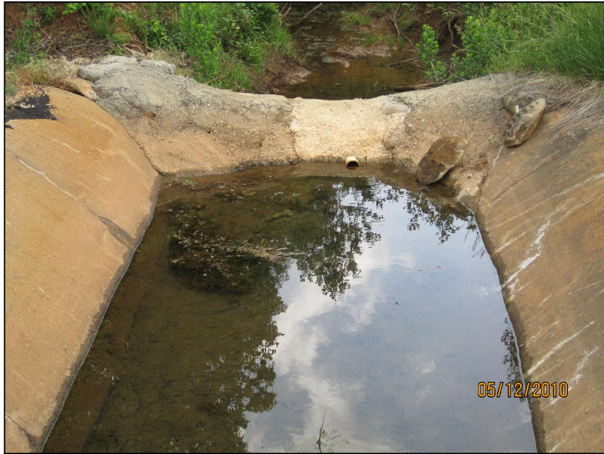
AP-31 DOWNSTREAM TOE OF EAST DIKE, LOOKING EAST AT BLANKET DRAIN OUTLET WITH 4-INCH DIAMETER PIPE
