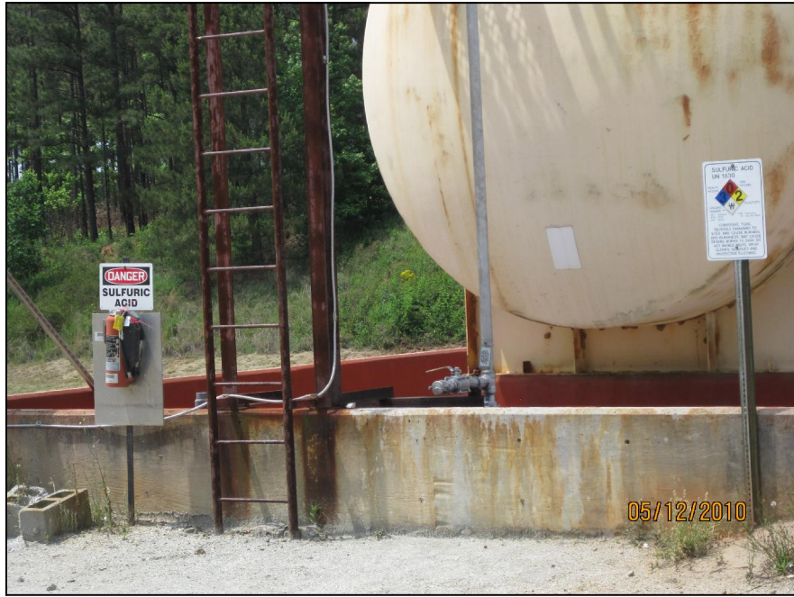
AP-37 SULFURIC ACID TANK FOR OUTLET TREATMENT
