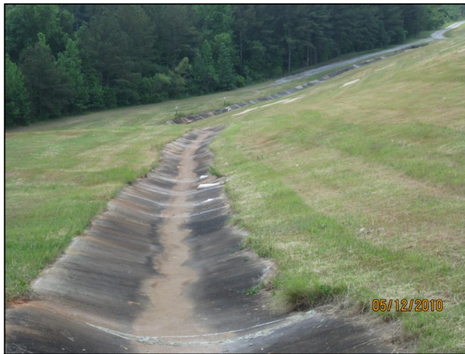
AP-34 DOWNSTREAM SLOPE OF EAST DIKE, LOOKING SOUTHEAST, TOP OF NORTH END OF ROAD AND BLANKET DRAIN CONCRETE DITCH
