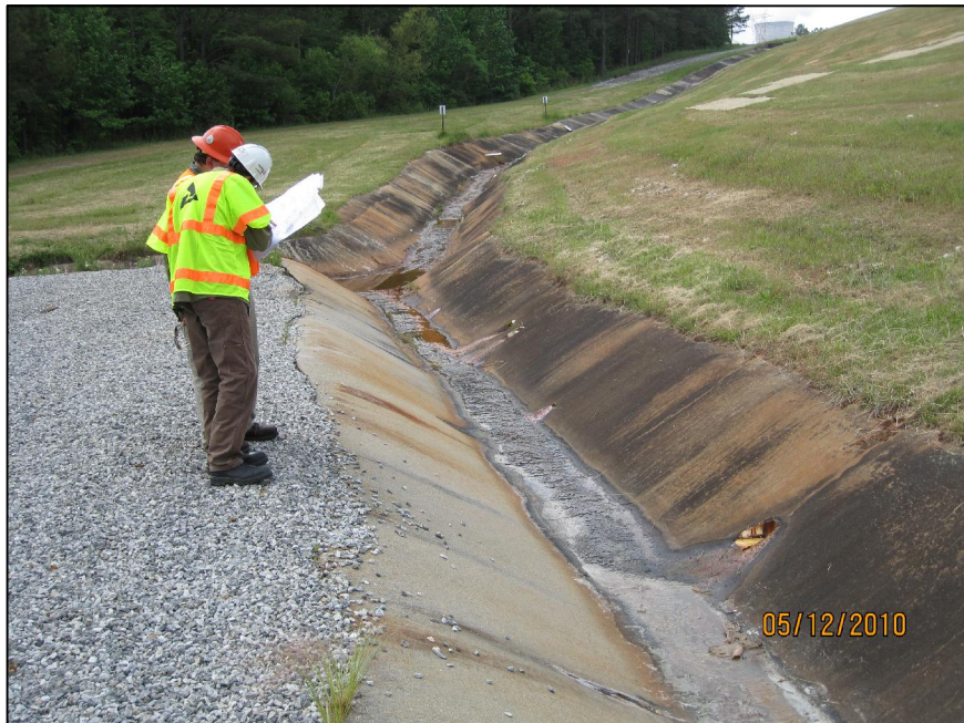
AP-32 DOWNSTREAM TOE OF EAST DIKE, LOOKING SOUTH AT FLOWING BLANKET DRAIN ON NORTH SIDE OF BLANKET DRAIN OUTLET
