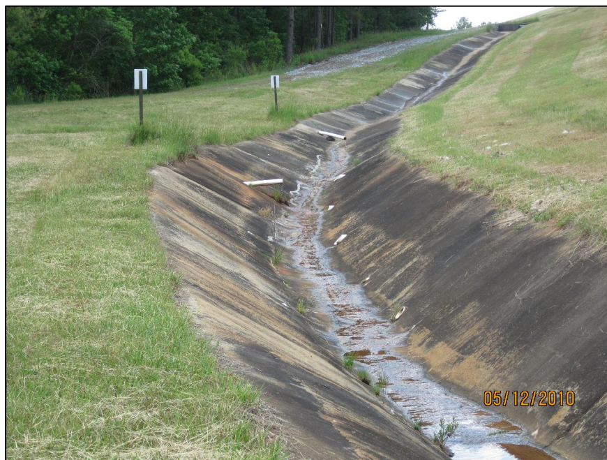
AP-30 DOWNSTREAM TOE OF EAST DIKE, LOOKING SOUTHWEST AT BLANKET DRAIN DITCH
