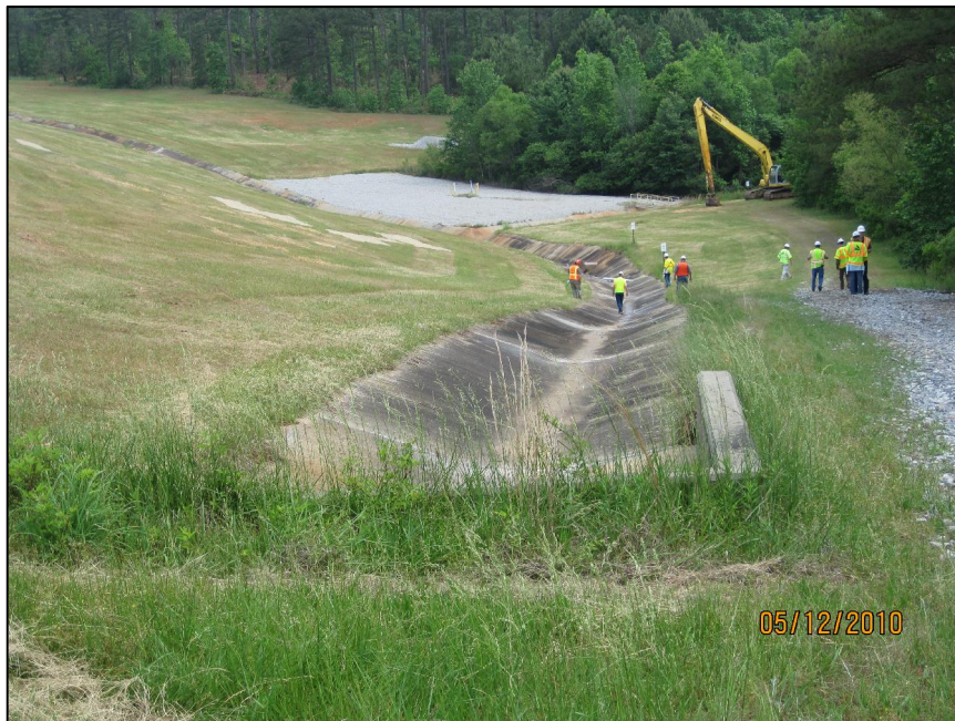
AP-26 DOWNSTREAM SLOPE OF EAST DIKE, LOOKING NORTHEAST, SOUTH END START OF SLOPE AND BLANKET DRAIN CONCRETE DITCH
