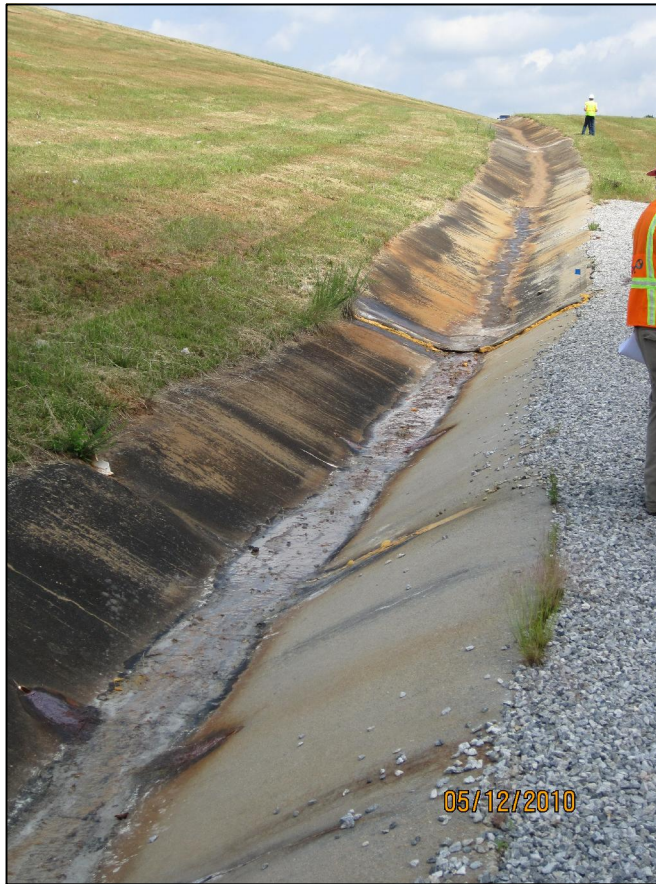
AP-33 DOWNSTREAM SLOPE OF EAST DIKE, LOOKING NORTH AT WATER SEEPING IN DITCH AND HEAVED JOINT ON NORTH SIDE OF BLANKET DRAIN OUTLET
