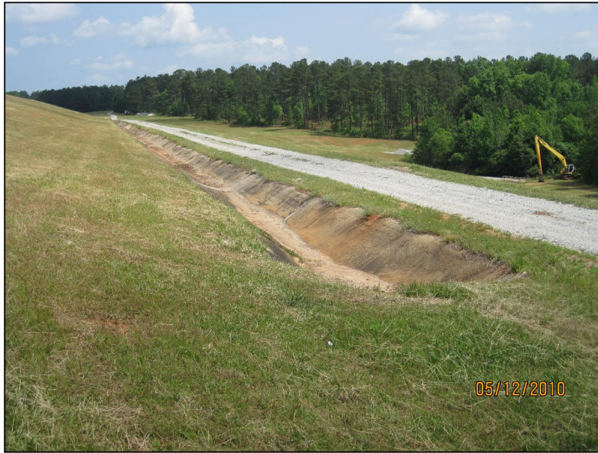
AP-25 DOWNSTREAM SLOPE OF EAST DIKE, LOOKING NORTH, END OF CONCRETE DITCH ABOVE GRAVEL ROAD
