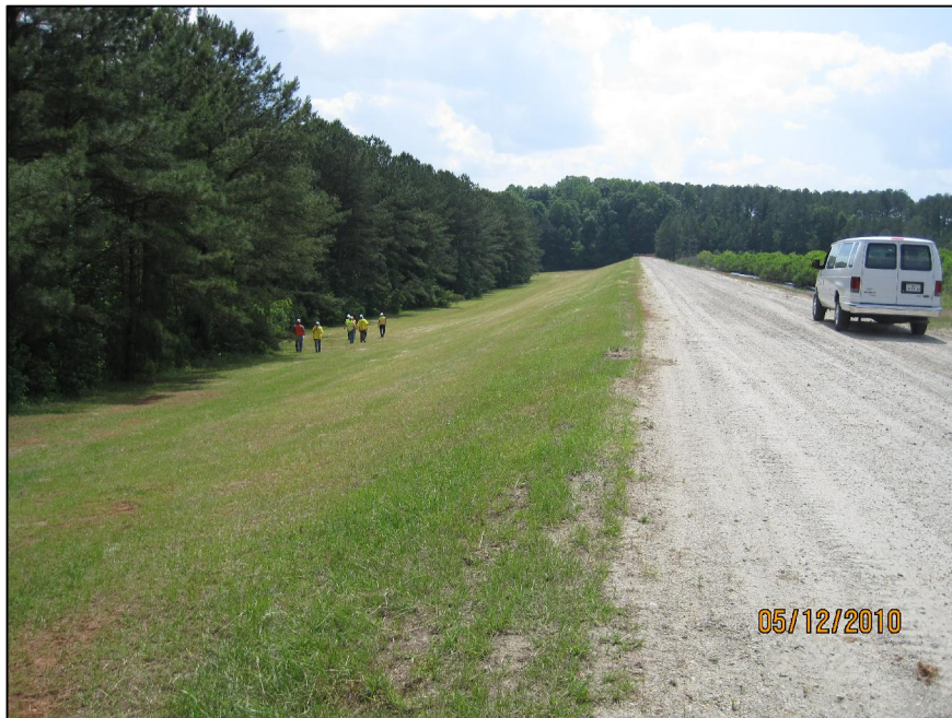
AP-46 CREST OF SOUTH DIKE, LOOKING WEST AT DOWNSTREAM SLOPE AND CREST
