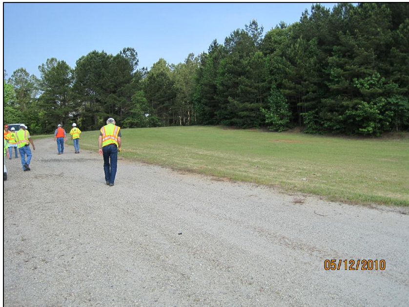
AP-12 CREST OF NORTH DIKE, LOOKING AT DOWNSTREAM SLOPE AT LEFT ABUTMENT TIE-IN
