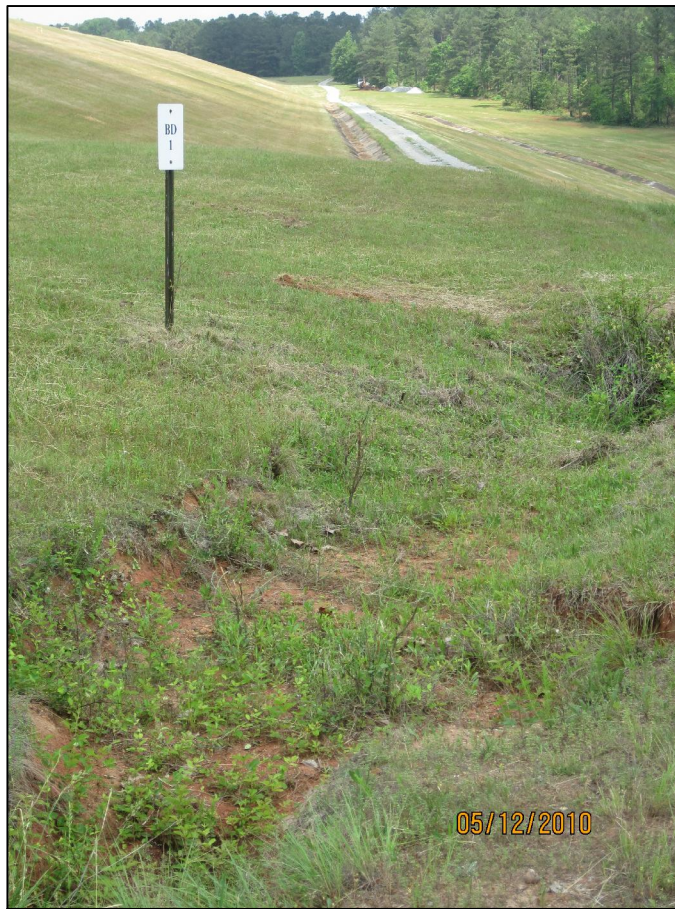
AP-35 DOWNSTREAM SLOPE OF EAST DIKE, LOOKING NORTHEAST AT BD-1 OUTLET, MINOR EROSION ABOVE THIS AREA
