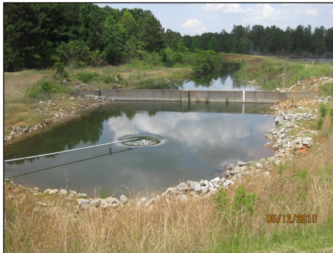
AP-36 ASH POND OUTLET WEIR AND DECANT PIPE (TREATMENT PIPE ABOVE DECANT)
