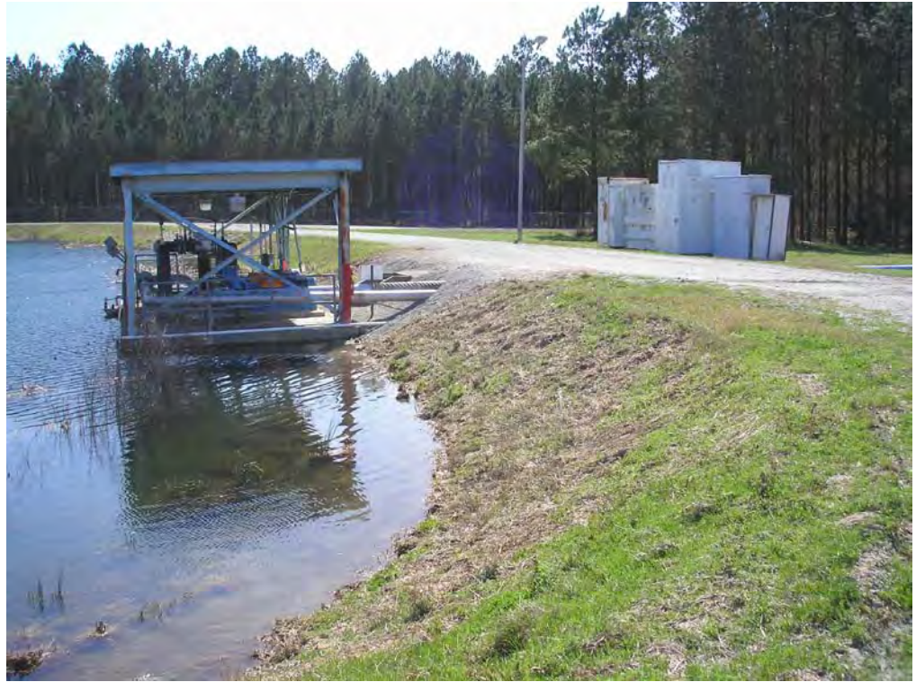
Figure 5.6.1-3 – Pumping Station to Recycle Water from CCR Impoundment Cell D to Plant.
