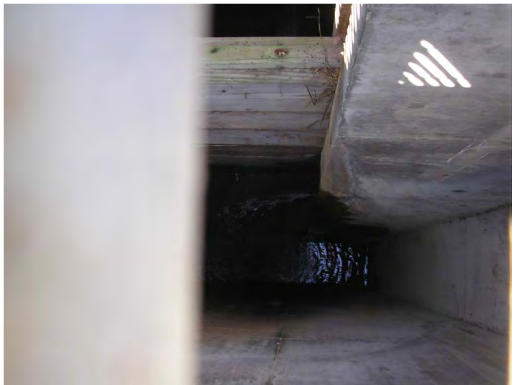
Figure 5.6.1-2: Primary Overflow Structure with Stop Logs in Place.
