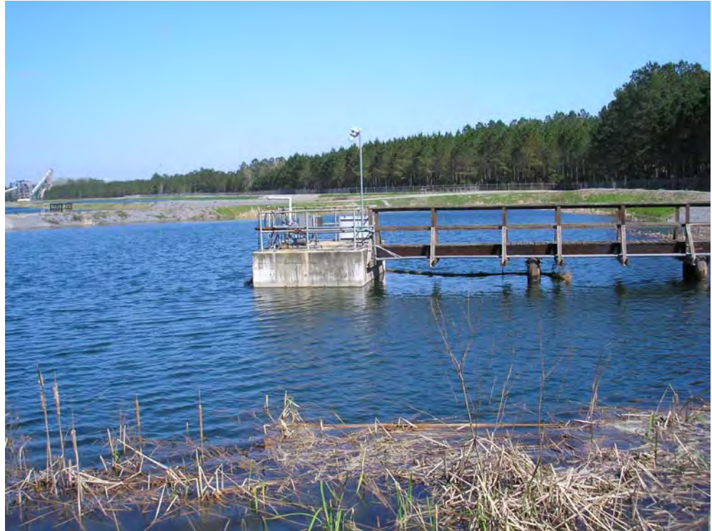
Figure 5.6.1-1 Primary Overflow Structure.
