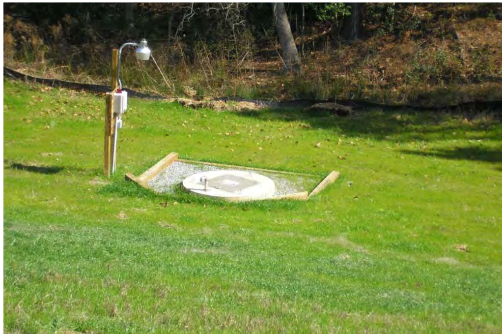
Figure 5.3.3-3 East Embankment Drainage System Sump
