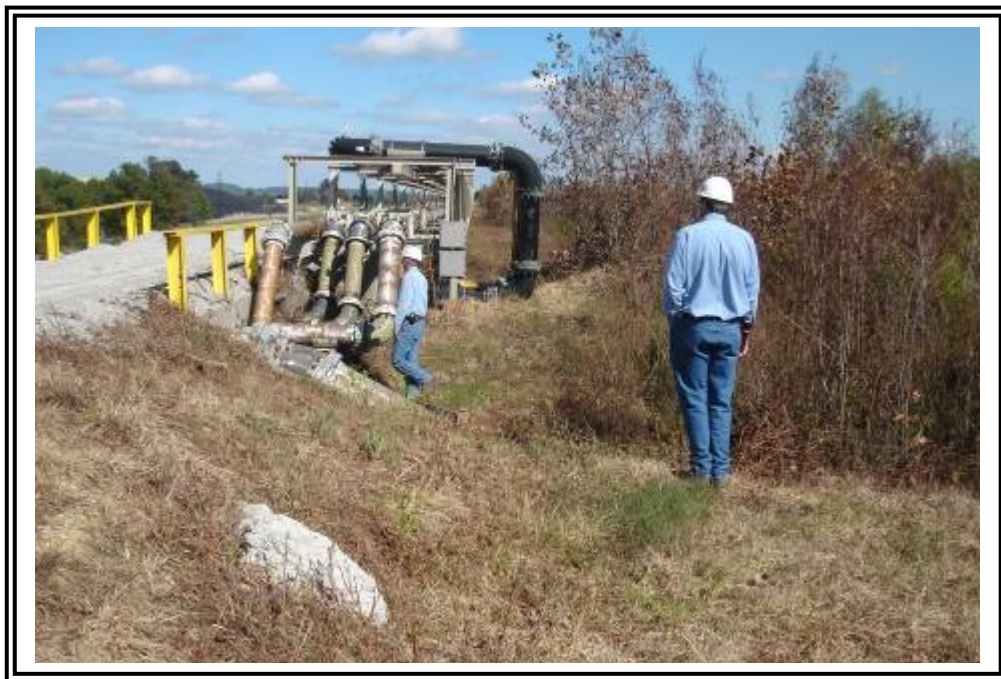
Upstream slope of ATB #1 north dike pipe racks for gypsum stacking facility. Note trees are growing on ash "not" dike.
