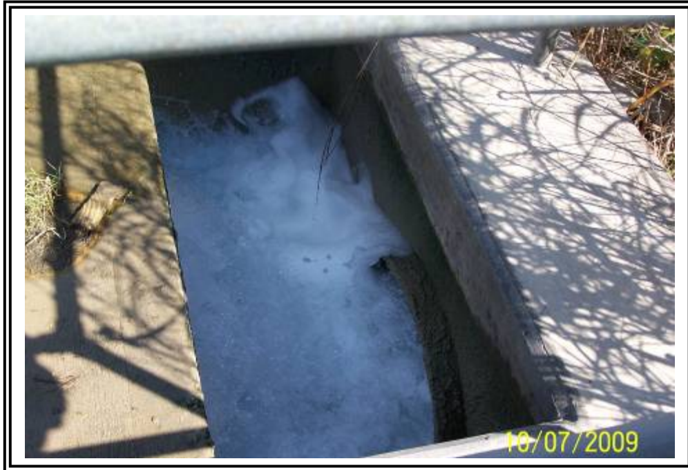
Discharge from ATB #2 near ATB #1. Discharges into structure with impact baffle.
