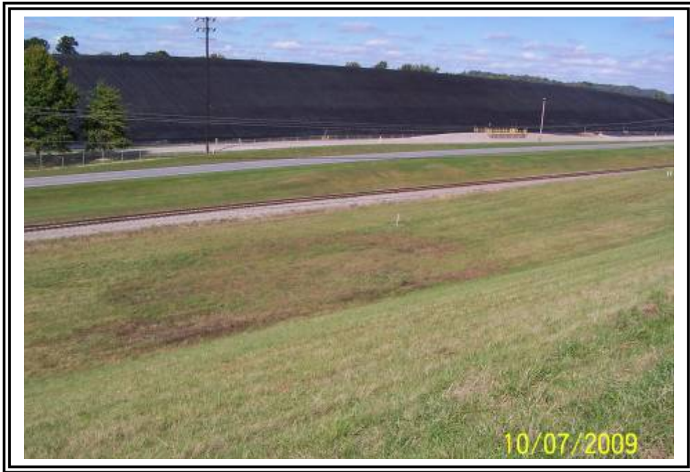
Area at mid point of ATB #1 north dike toe appeared wet. Area firm when probed, Kentucky Utilities indicated area may be where a water line burst and was repaired.
