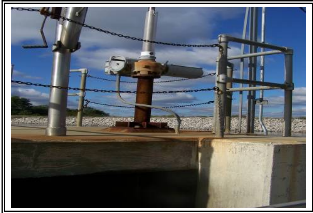
Outlet structure equipped with gates to close outlet flow from discharge pipe.
