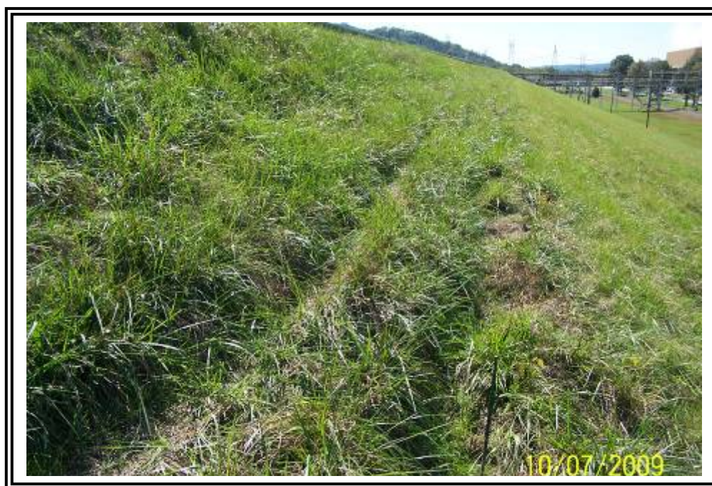
Tire ruts from mower on over steepened area.
