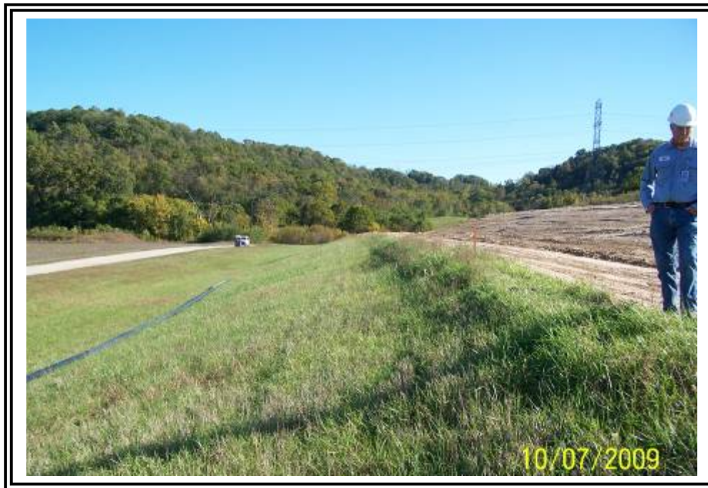
Over steepening at crest of east side of gypsum stacking facility starter dike, looking south.
