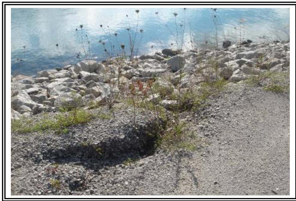
Erosion rill on upstream slope.
