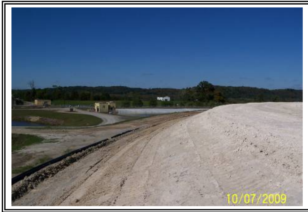
Downstream slope of northwest corner of gypsum stacking facility dike above starter dike (under construction from dewatered gypsum).
