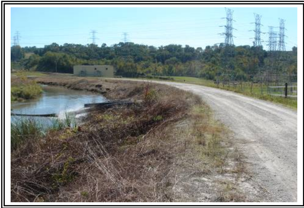
Upstream slope at northwest corner of ATB #1 looking southwest.
