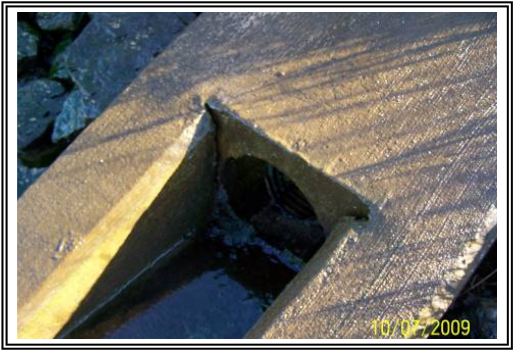
Toe drain at northeast corner of ATB #1. No apparent flow, concrete is wet from splash from outlet pipe.
