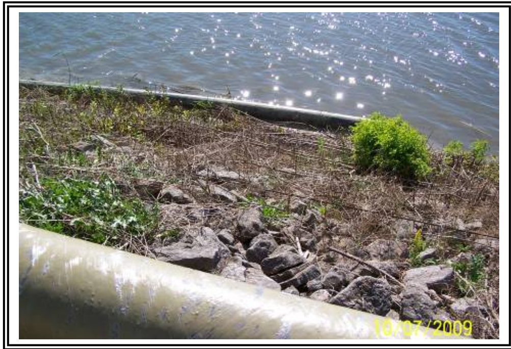
Upstream slope of ATB #1 east dike. Rip rap has been placed to fill areas of erosion.
