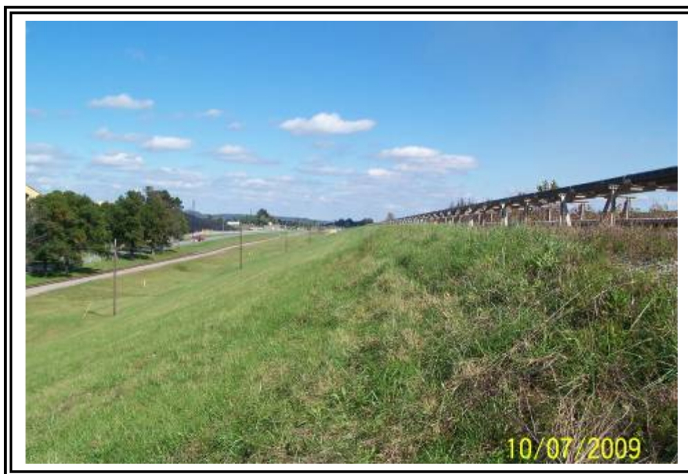
Downstream slope of ATB #1 north dike. Note over steepening adjacent to crest, looking east.
