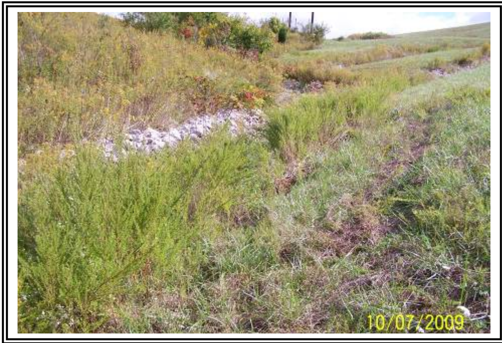
Taller weeds along drainage swale at toe.
