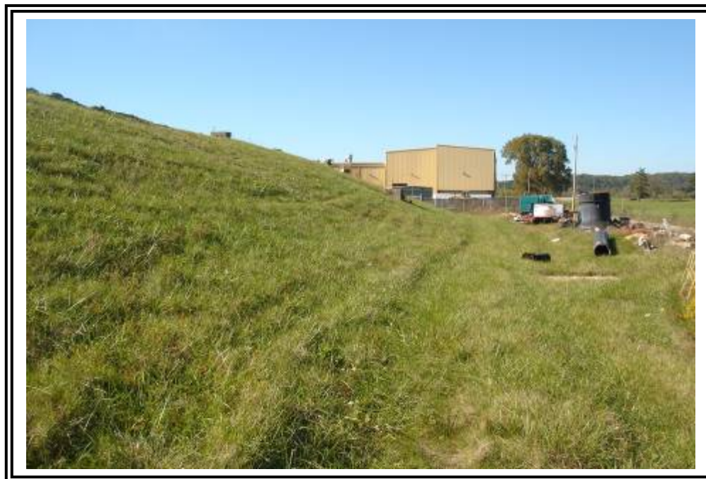
Downstream slope of east side of gypsum stacking facility starter dike, looking north.
