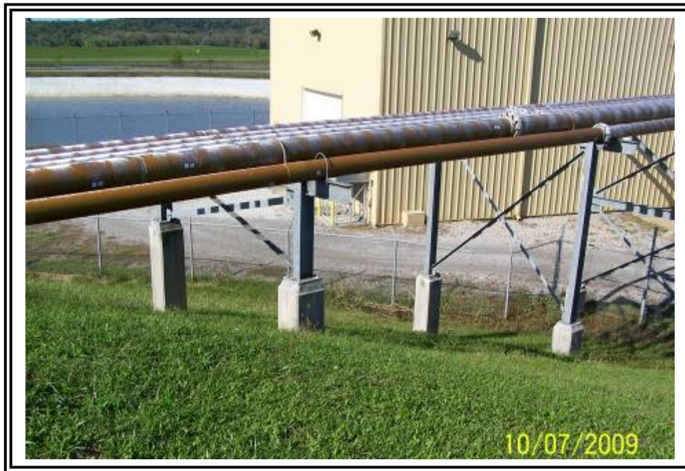
Pipe rack diverting gypsum to reuse facility on northeast corner of the gypsum stacking facility starter dike.
