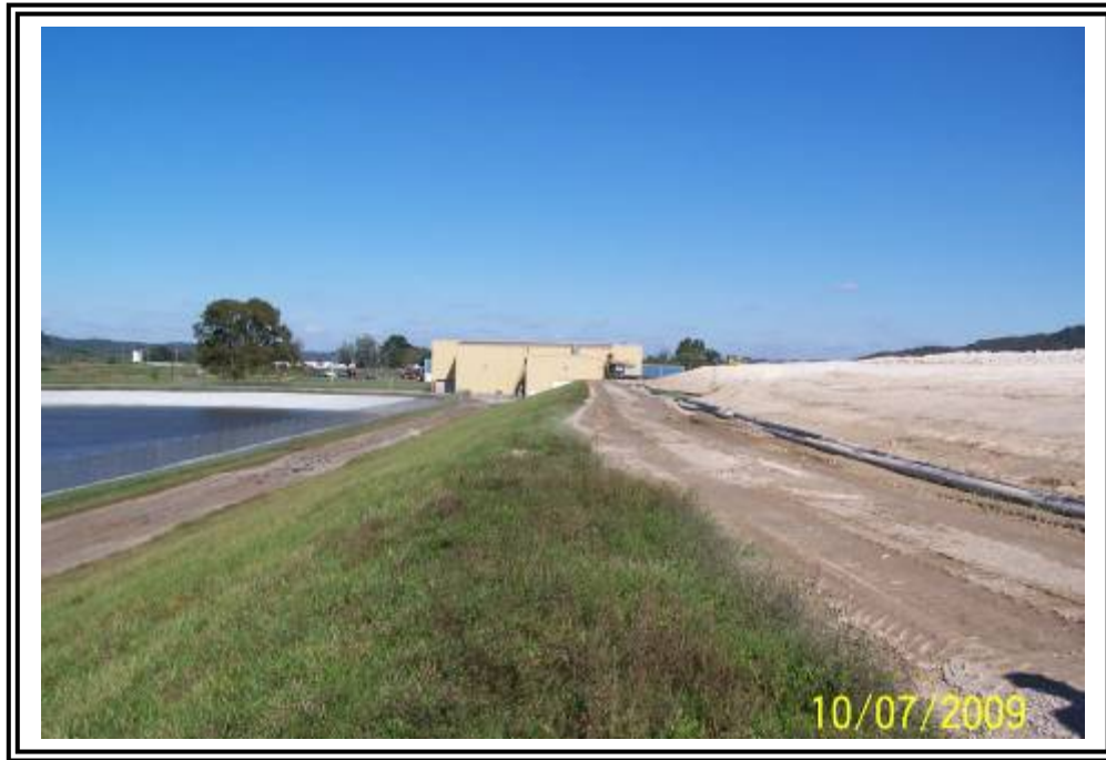
Crest of starter dike, north side of gypsum stacking facility, looking east.
