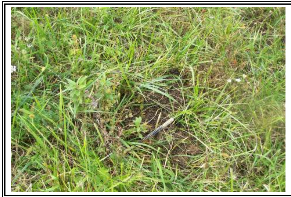
Small rodent hole on bench in secondary drainage fill section about 18 inches deep.
