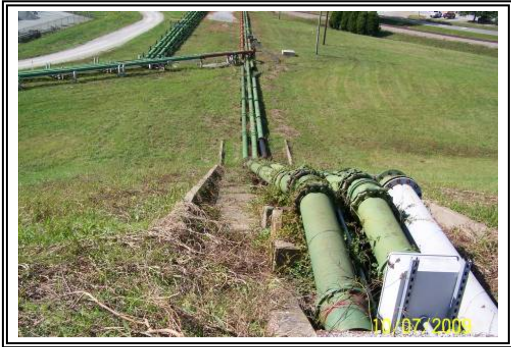
Utility corridor at northwest corner of ATB #1.
