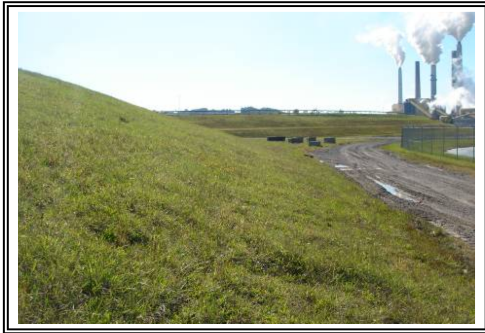
Depressions at toe of north side of starter dike of gypsum stacking facility, looking west.
