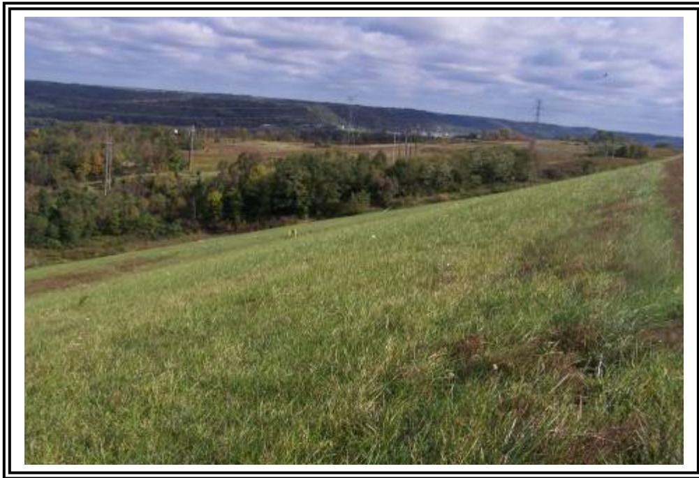
Upper portion of downstream slope of ATB #2 looking northeast. Instrumentation marked with yellow bollards, horizontal benched in main section of Dike at 50 vertical foot increments.
