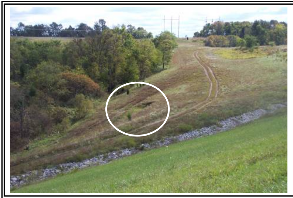
Slump in natural slope near the east abutment of ATB #2.
