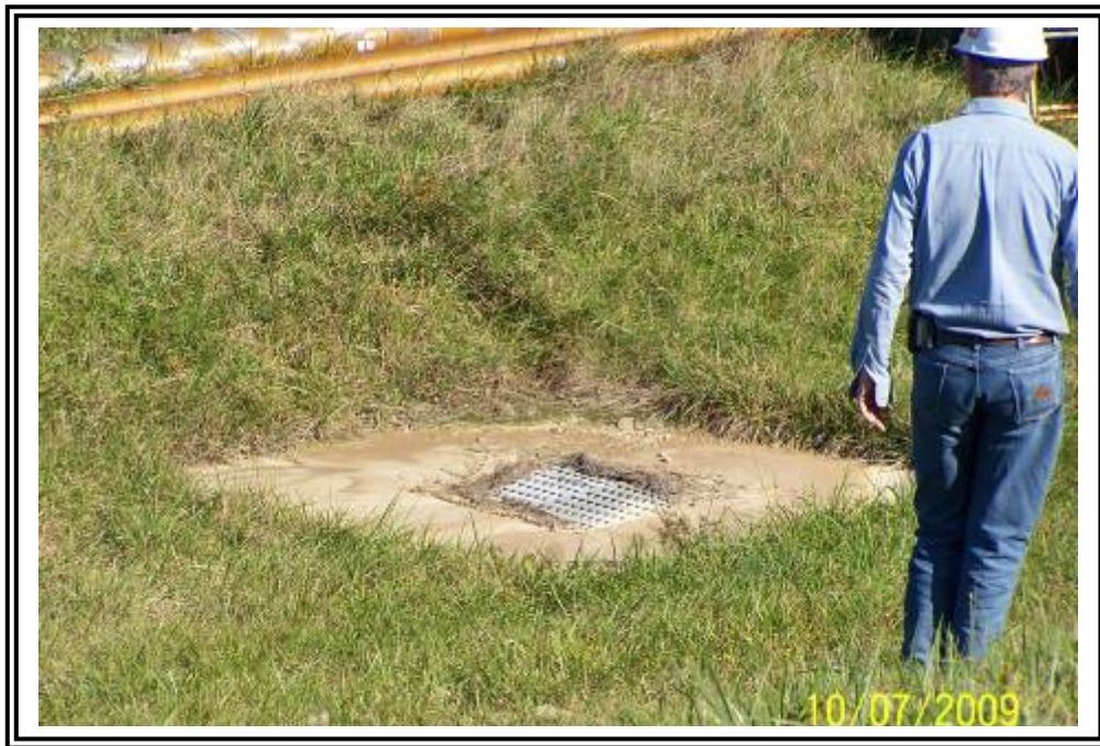
Surface drainage system on east side of gypsum stacking facility starter dike.
