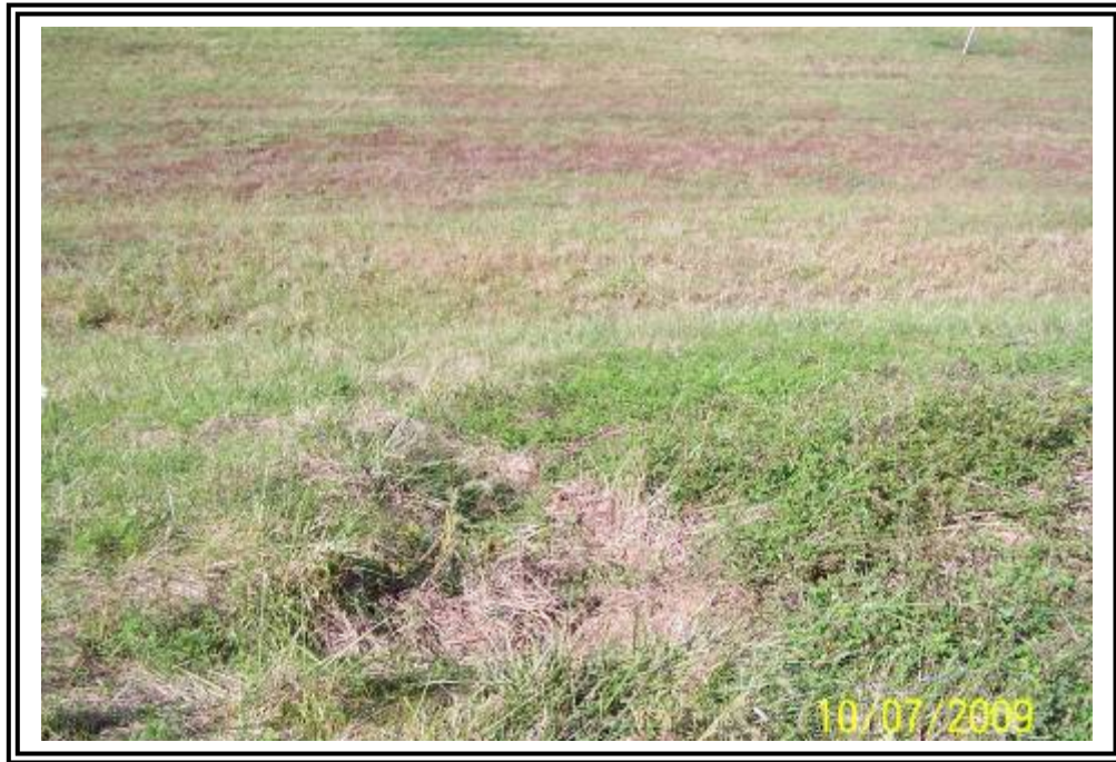
Depression in bench near northeast corner of ATB #1 dike.
