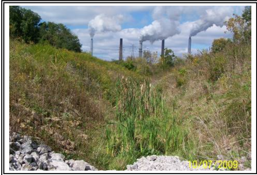
Channel below toe of main fill. No discharge, standing water and wetland plants observed likely from seepage/toe drain outlet.
