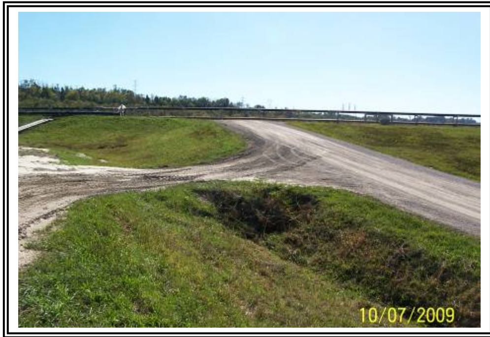
Drainage swale at northwest corner of gypsum stacking facility dike, looking southwest. ATB#1 dike beyond.
