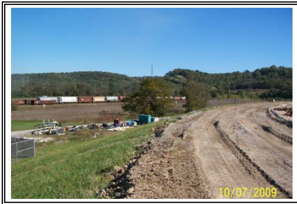
Crest of starter dike at northeast corner of gypsum stacking facility (under construction).
