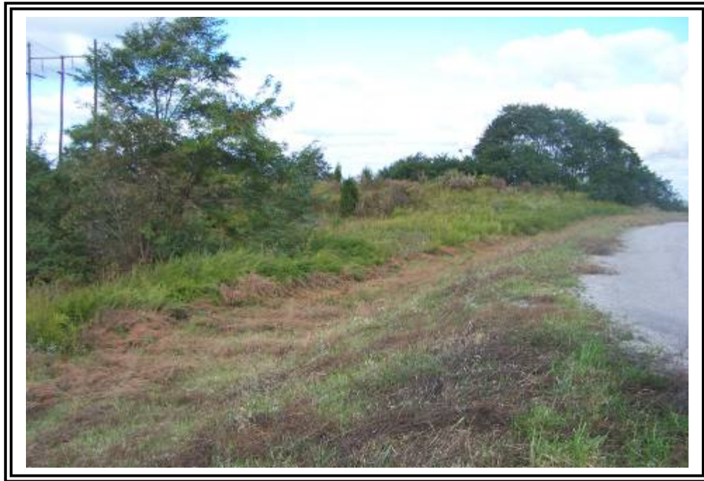
Downstream slope west end of dike looking north. Taller grass is on natural ground.
