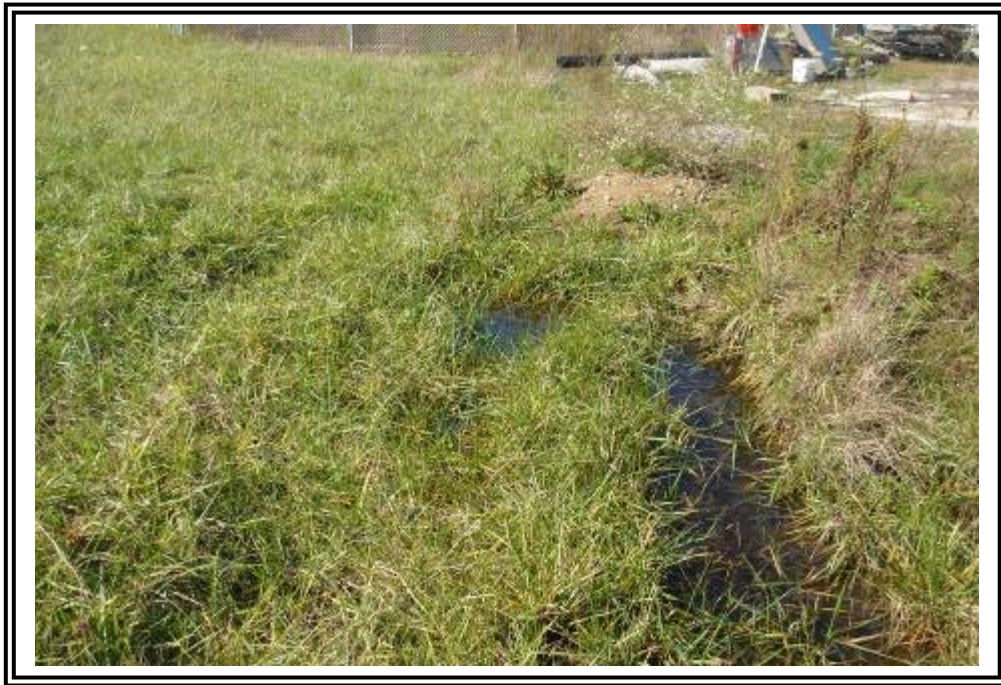
Standing water at the toe along the east side of the gypsum stacking facility starter dike. Ground is firm, appears to be surface water drainage.
