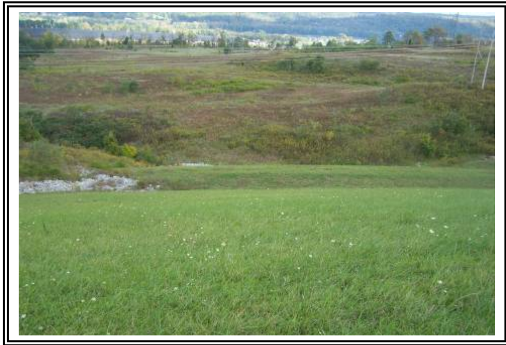
Downstream slope of ATB #2 just east of eastern knoll looking northeast.
