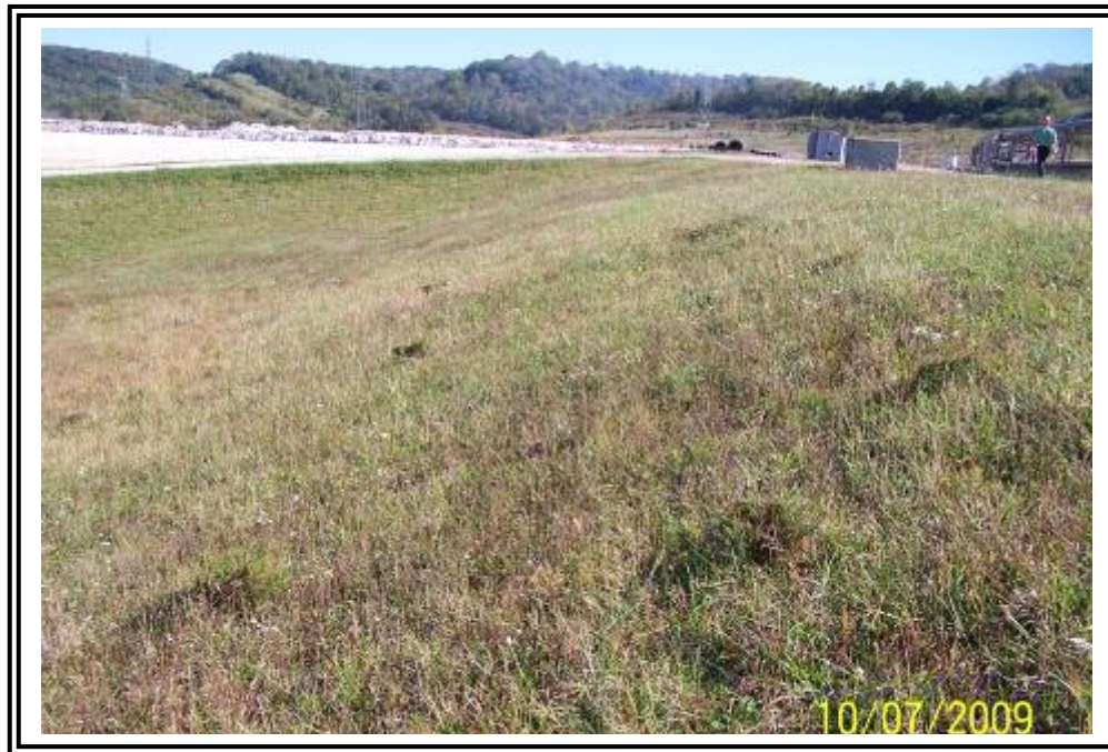
Downstream slope at north end of ATB #1 east dike. The east dike is now shared with the gypsum stacking facility.
