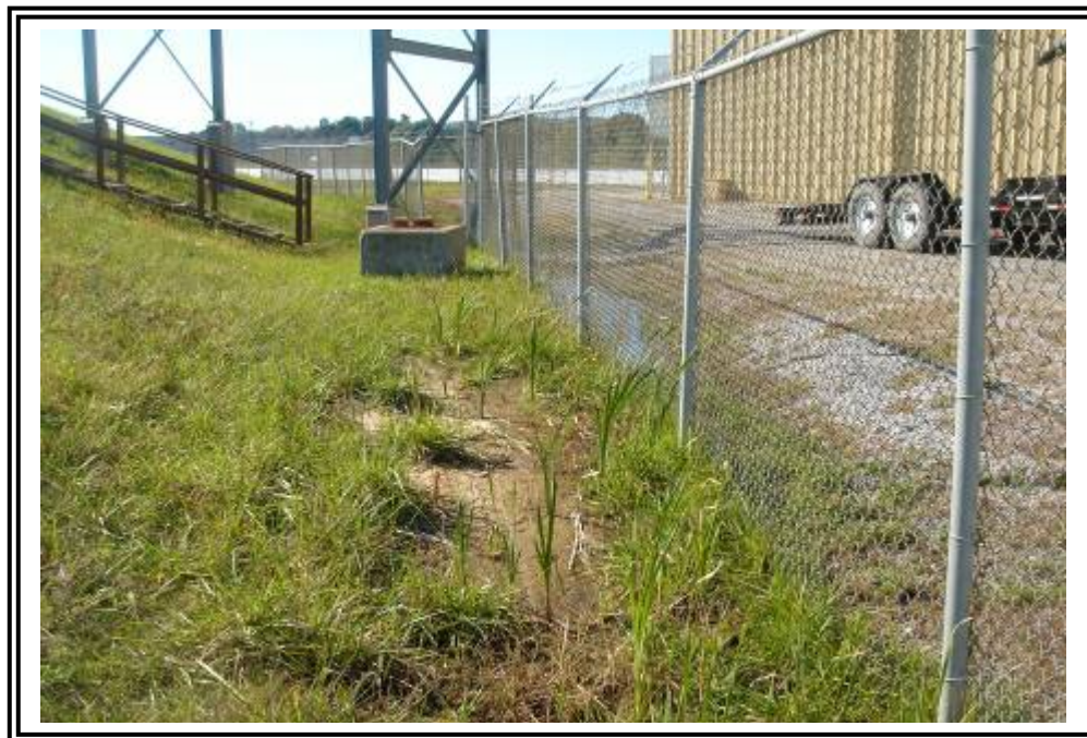
Standing water at toe at northeast corner of gypsum stacking facility starter dike. Appears to be surface drainage water.
