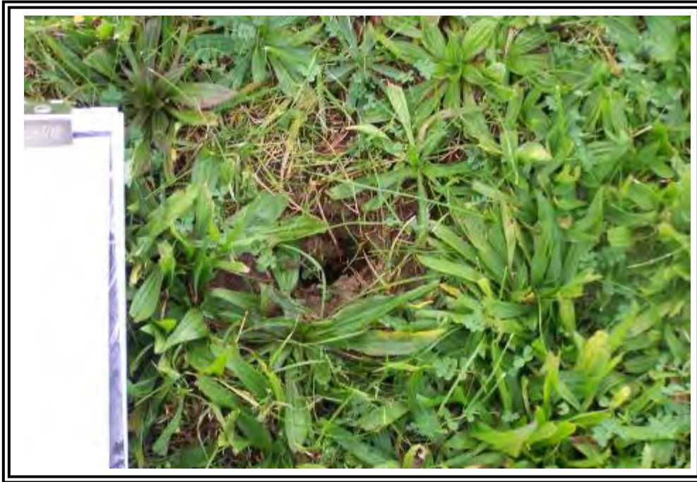
Small rodent hole on ATB north dike.
