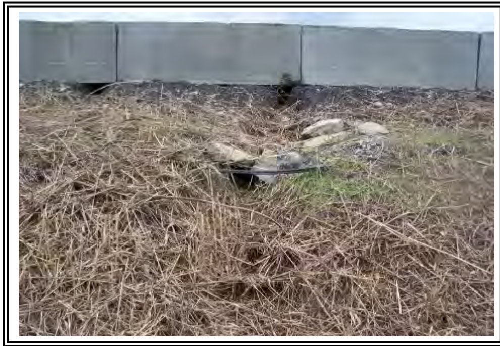
Erosion rills under concrete barriers at crest of south dike adjacent to the E-Pond.
