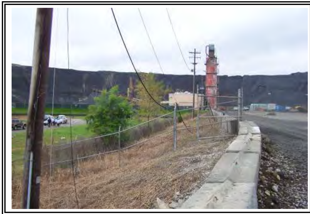
Downstream slope and crest of west end of ATB south dike where adjacent to the E-Pond, looking west.
