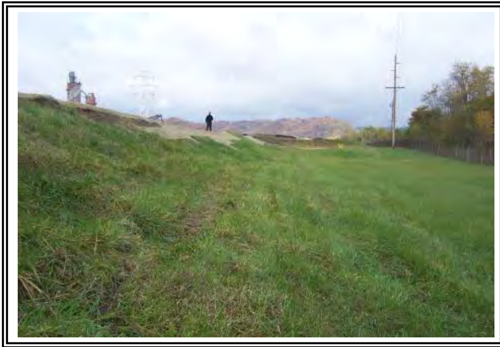
Downstream slope of north dike at Basin/ Dead Storage Pond looking west.
