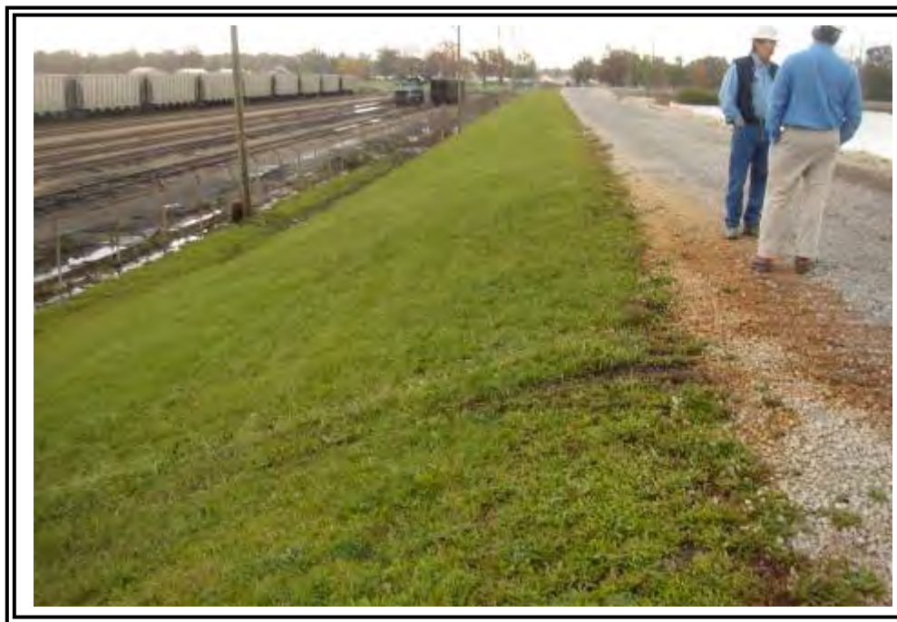
Slight erosion rill from crest on ATB north dike looking east.
