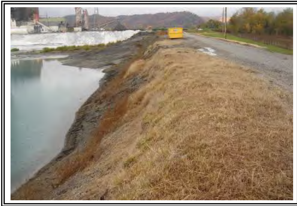
Upstream slope of north dike at Basin/ Dead Storage Pond looking west.
