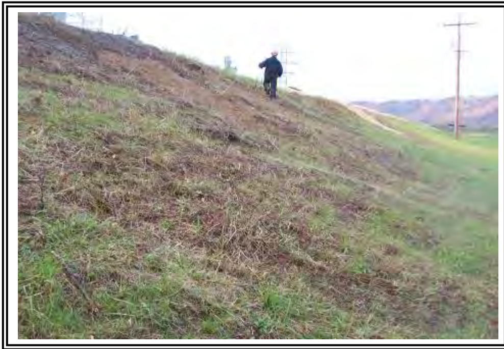
Irregularity on north dike at Basin/ Dead Storage Pond. Combination of surface slumps, erosion rills, etc. Probes soft to about 9" then firm.
