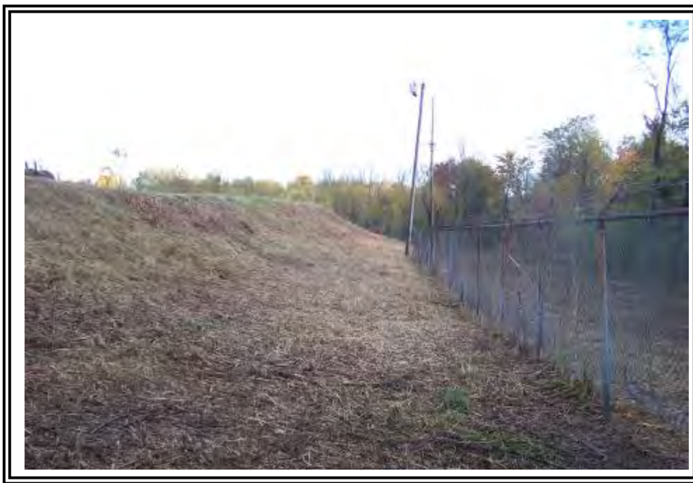
Downstream slope of east dike at Basin/ Dead Storage Pond at toe looking north.
