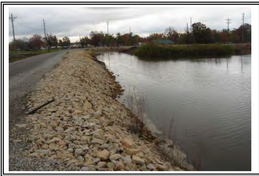
Upstream slope and crest of ATB north dike looking east near east corner.
