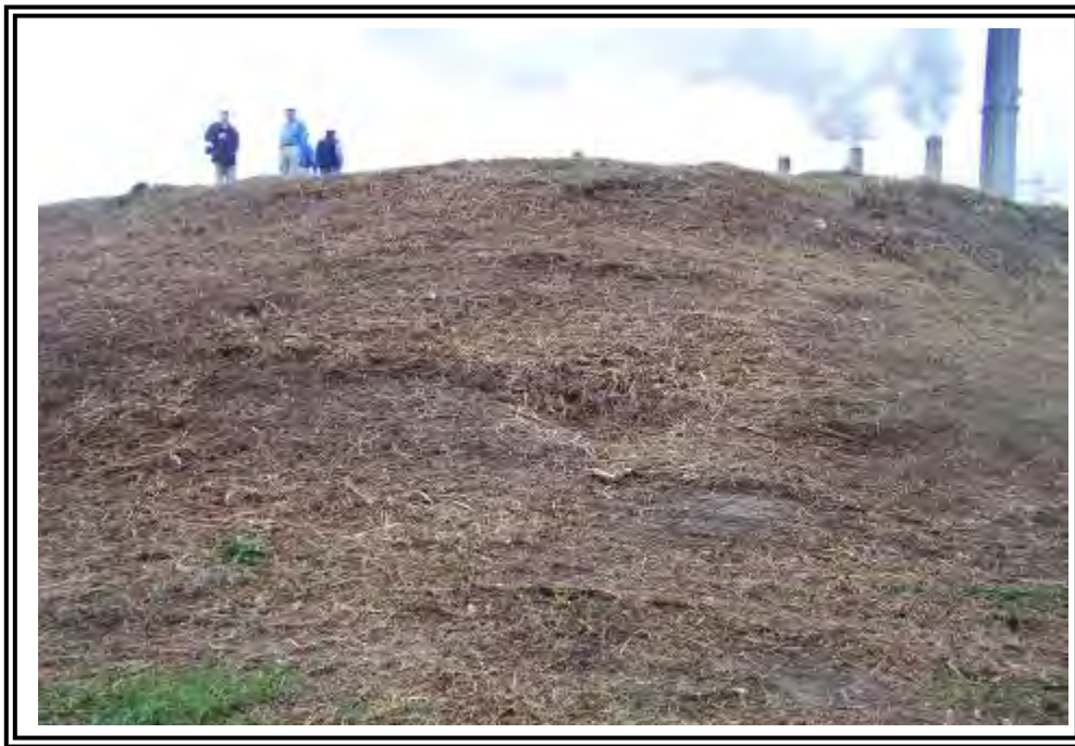
Depressions and irregular grading at northeast corner of Basin/ Dead storage pond dike.
