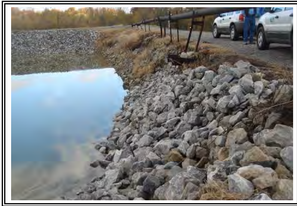
Upstream slope of east dike at Basin/ Dead Storage Pond looking north along south cell.
