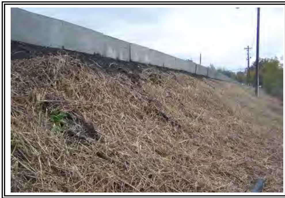
South dike of ATB adjacent to the E- Pond is quite steep. A January 2010 survey indicates it is at 2H:1V.
