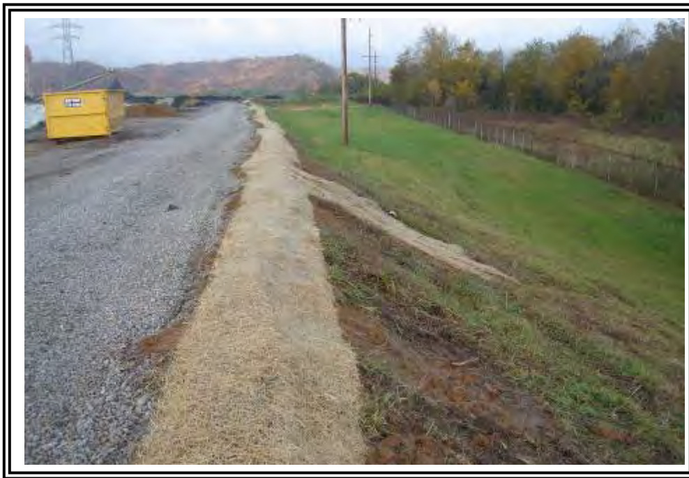
Recent regrading along crest of north dike of Basin/ Dead Storage Pond to improve stormwater control.
