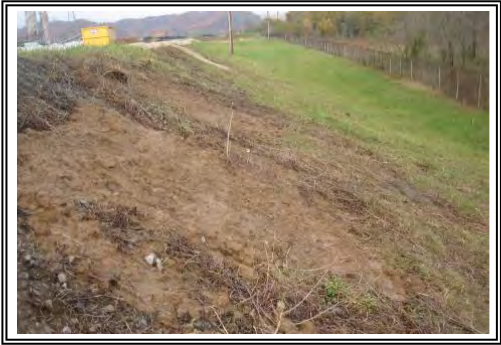
Repair area at north dike of Basin/ Dead Storage Pond not yet reseeded.
