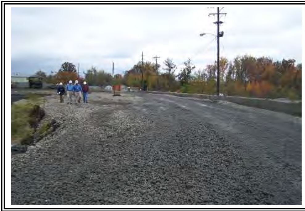
E-Pond (left of people) is excavated within previously deposited ash. Original ATB south dike and ash create south side of the impoundment.
