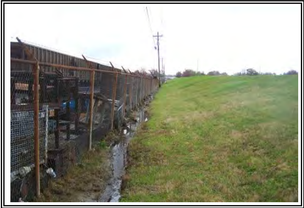
Downstream slope of north dike at ATB looking east. Poor drainage results in standing water at the toe of this dike. E.ON U.S. is working with a consultant to re-grade this area for better drainage.
