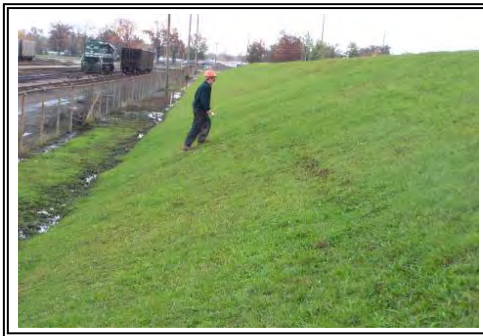
East end of north dike at ATB looking east. Mower ruts, and toe erosion from stormwater were observed.
