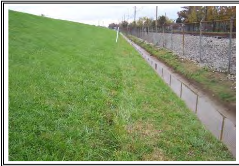
Downstream slope of ATB south dike looking east. White marker indicates locations of gas line. Slight depression appears to be over the pipe alignment along the south dike.
