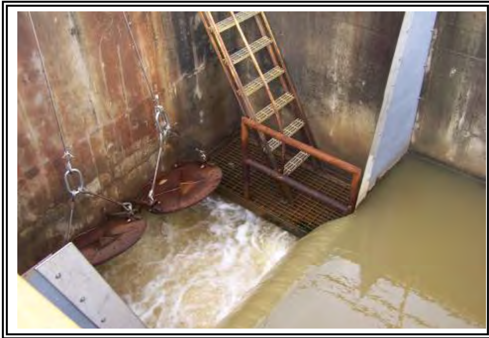
ATB discharge to KYPDES permitted outfall. Pipes (beyond flap gates) discharges at Ohio River.
