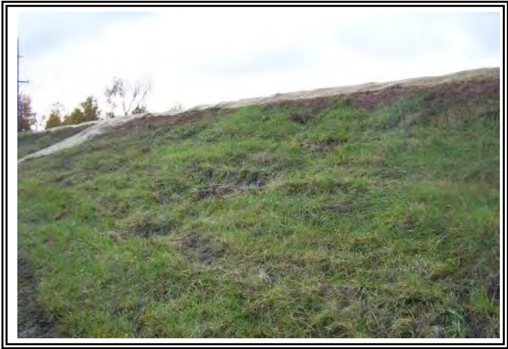
Tire ruts in north dike of Basin/ Dead Storage Pond.
