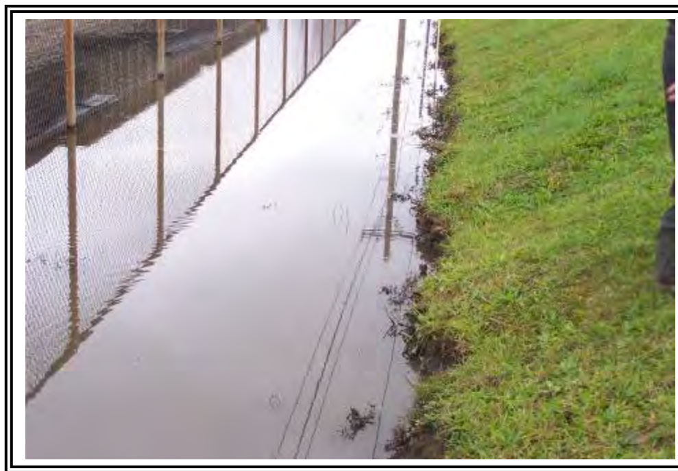
Close up of toe erosion on ATB north dike.
