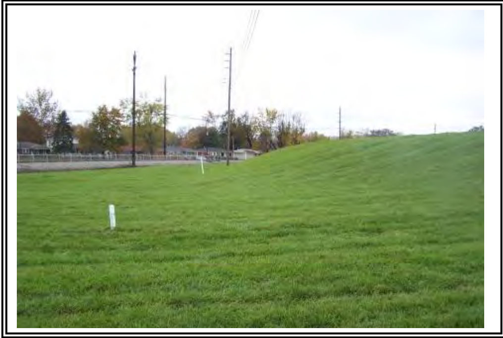
Downstream slope of ATB east dike looking south. The area at the toe was raised 1 to 2 feet in summer 2009 and sod placed to prevent stormwater pooling in this area. White markers indicate the location of a high pressure gas line installed in 2005.
