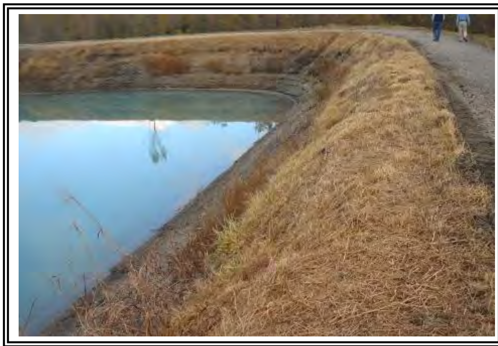
Upstream slope of east dike at Basin/ Dead Storage Pond looking north along north cell.
