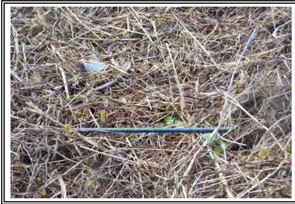
Erosion rill about 6 inches deep, 1.5 feet wide on east dike at Basin/ Dead Storage Pond.
