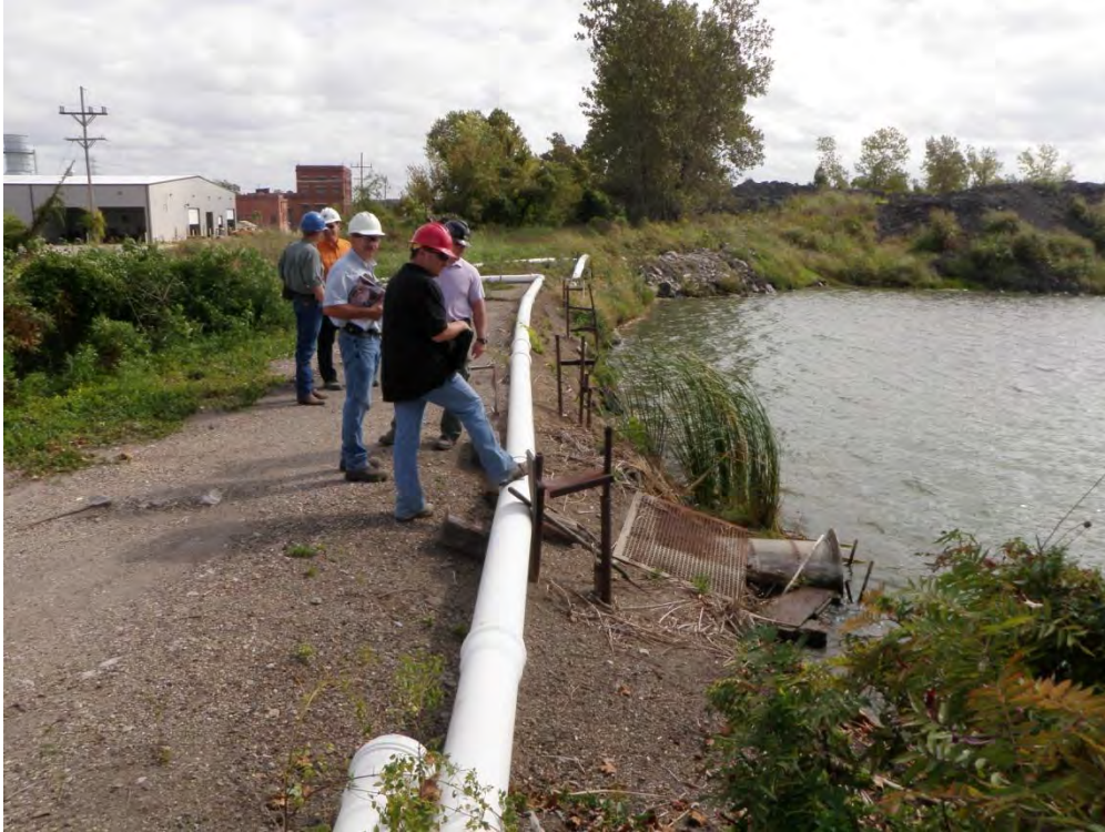
Photo 15: Outlet pipe in East Cell and PVC intake pipes located along north perimeter dike.
