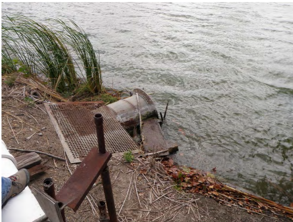
Photo 14: Riveted steel outlet pipe located in northwest corner of the East Cell (note trashrack above pipe).
