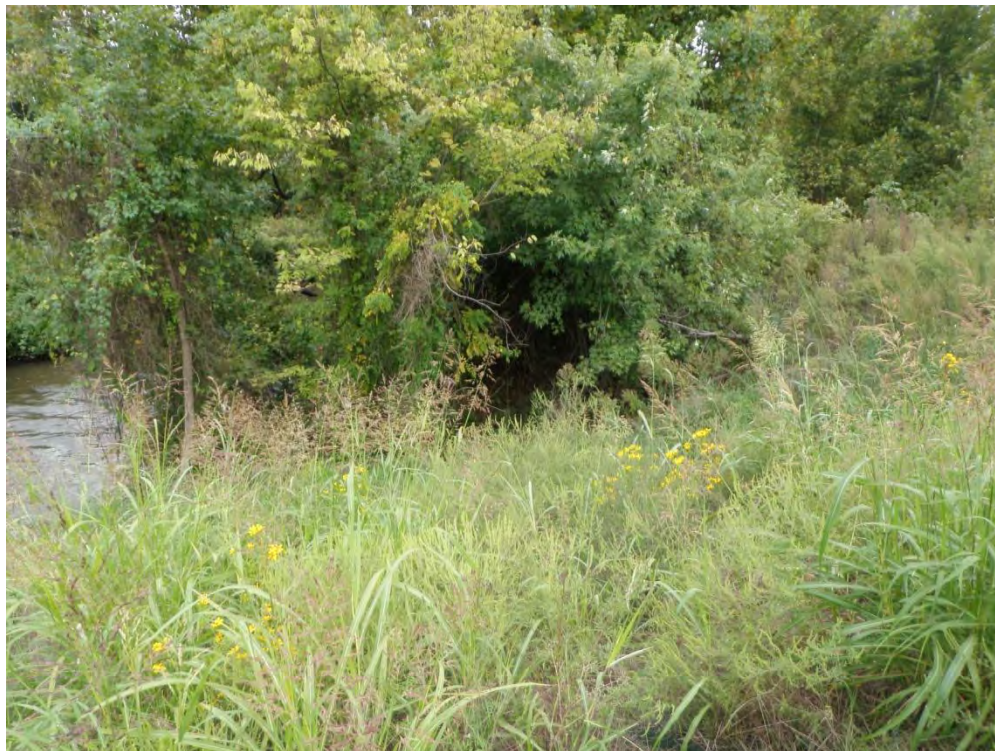
Photo 3: Heavy vegetation in downstream slope of east perimeter dike, East Cell.
