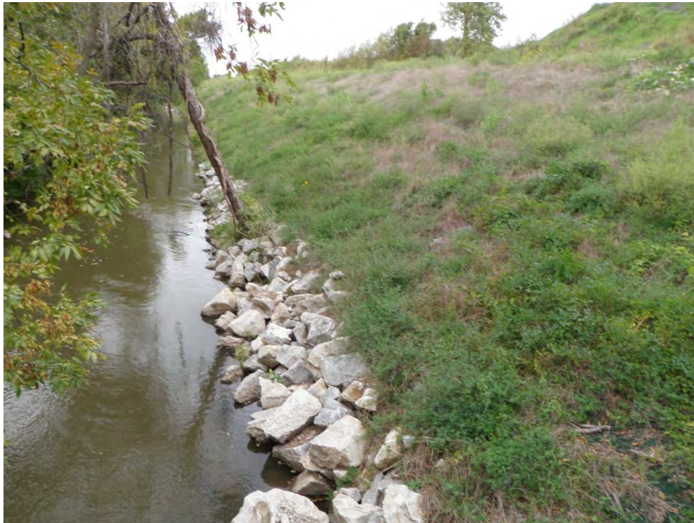
Photo 1: Riprap at downstream toe of the perimeter dike in the cooling water discharge channel.
