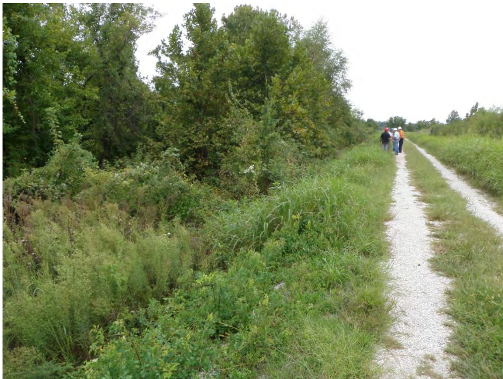
Photo 2: Heavy vegetation and large trees in downstream slope of east perimeter dike, East Cell.
