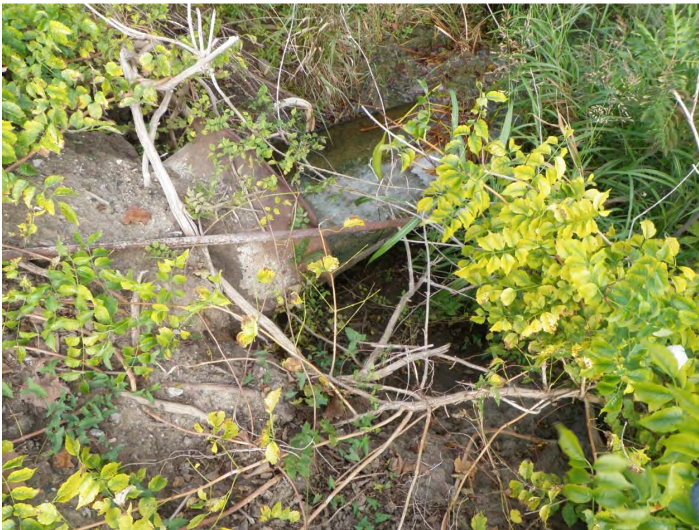
Photo 16: Discharge from outlet pipe.
