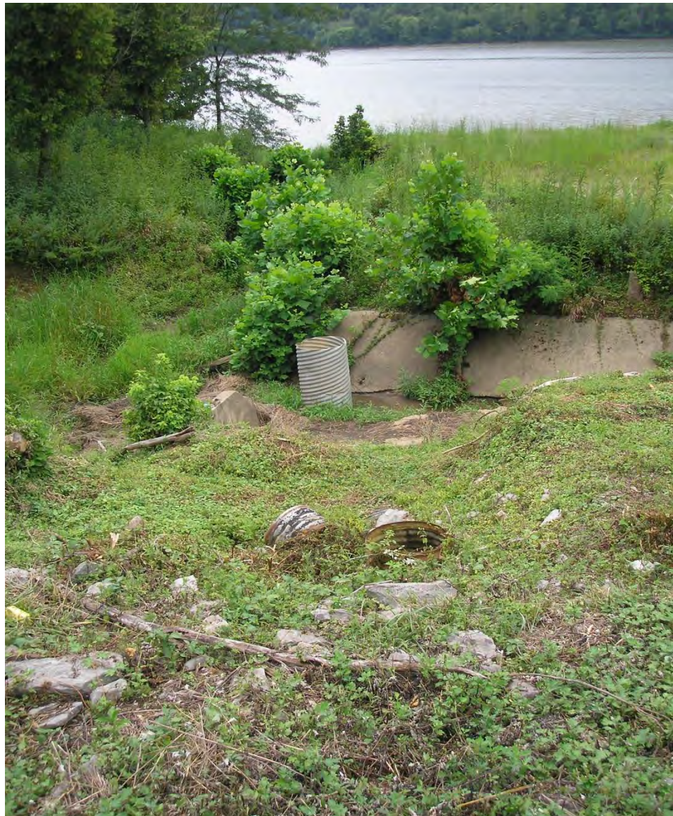
Figure 5.3.2-1: Photo of Primary Spillway Outlet Pipe Vents
