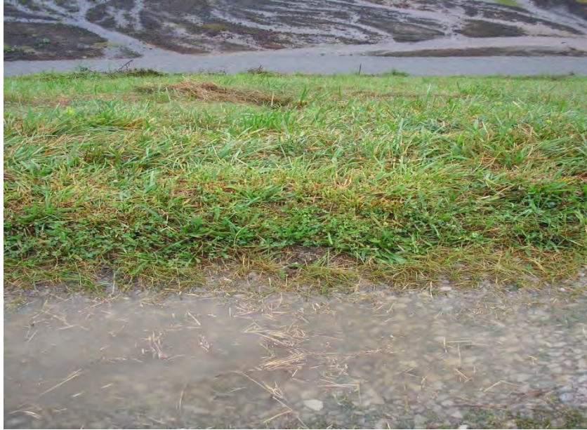
Figure 5.2.1-2: Water Ponding in Small Depression in Gravel Travel Track along Embankment Crest.
