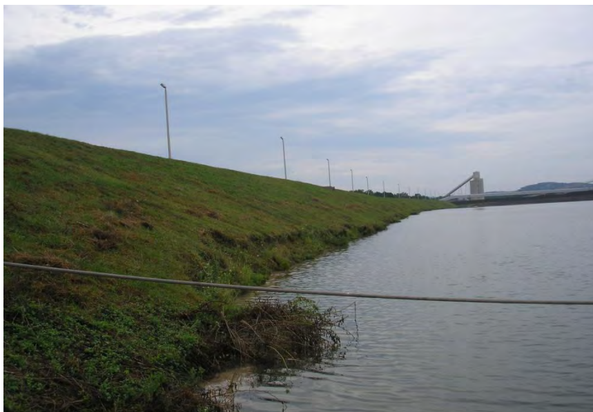
Figure 5.2.2-6: Up-gradient Embankment Toe Wave Erosion near Primary Spillway Structure
