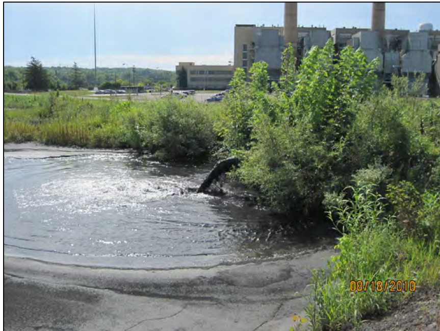
E-4 INLET PIPES FROM PLANT TO EAST PRIMARY SETTLING POND LOCATED AT SOUTHWEST CORNER OF POND
