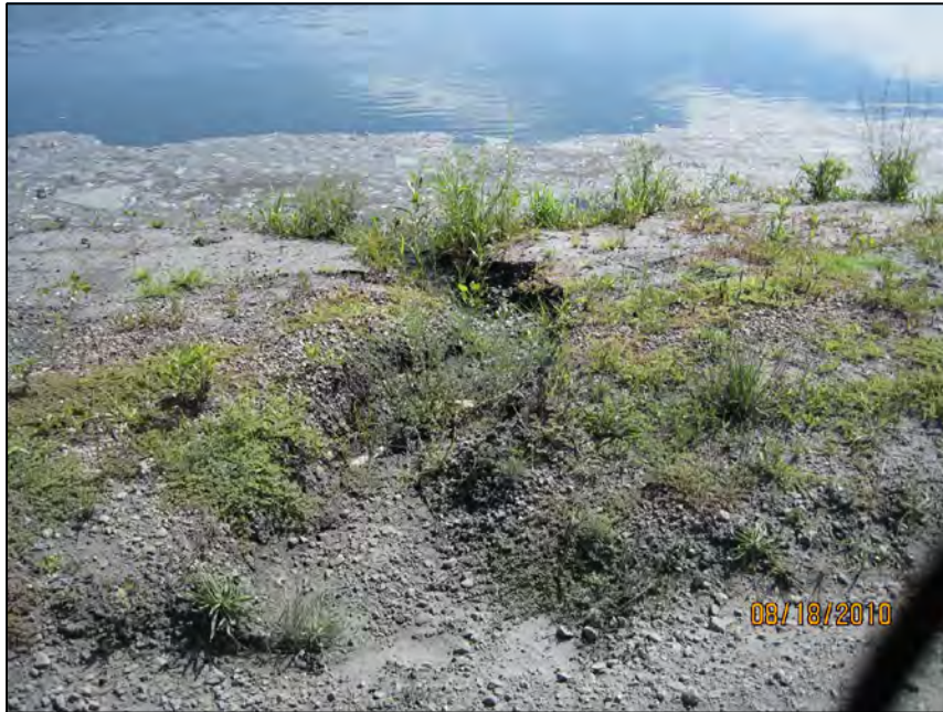
E-17 EROSION RILL ALONG WESTERN INTERIOR SLOPE
