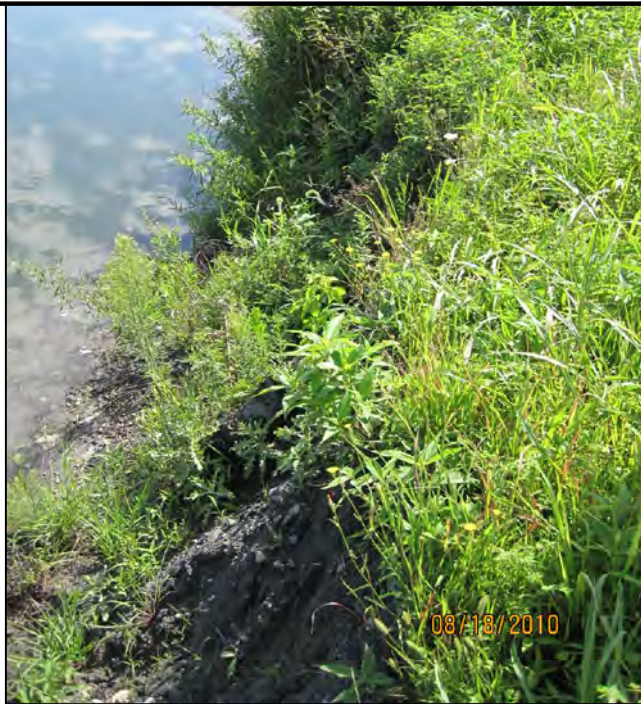
W-11 ERODED SOUTHERN INTERIOR SLOPES
