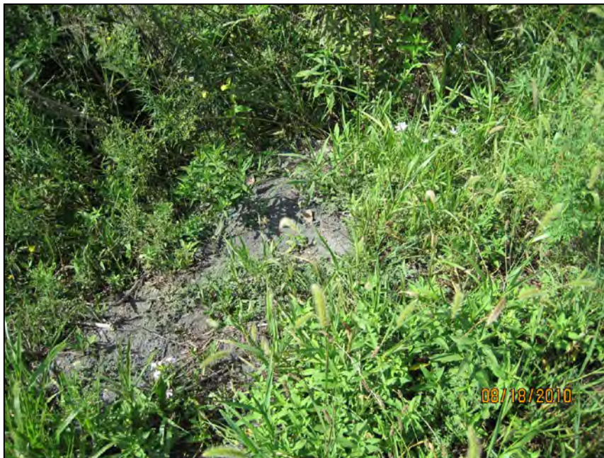
W-12 ASH NOTED ON SOUTHERN DOWNSTREAM SLOPE
