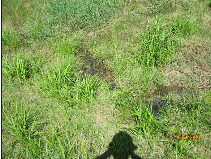
E-11 WET AREA ALONG SOUTHERN DOWNSTREAM TOE
