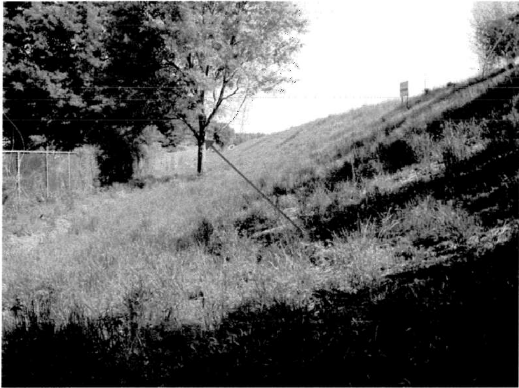
Photo 7 – Tree on Toe of West Dike
