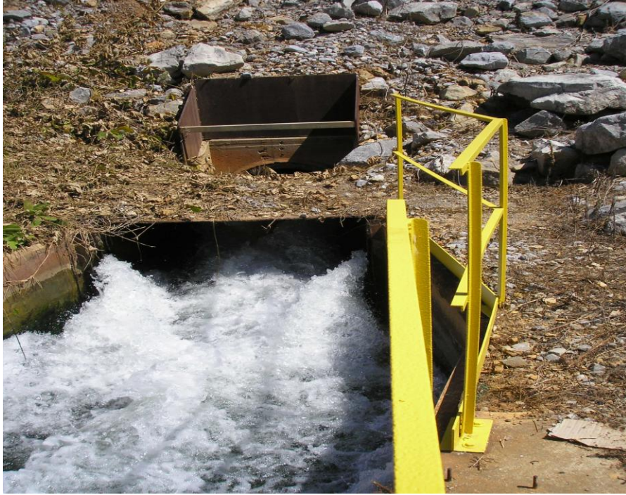
Figure 5.3.2-1 Photo Showing Water Discharge from Outlet Pipe.
