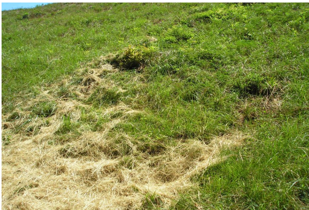
Figure 5.2.3-6 Photo Shows Small Area of Sloughing on West Dike Downstream Slope.
