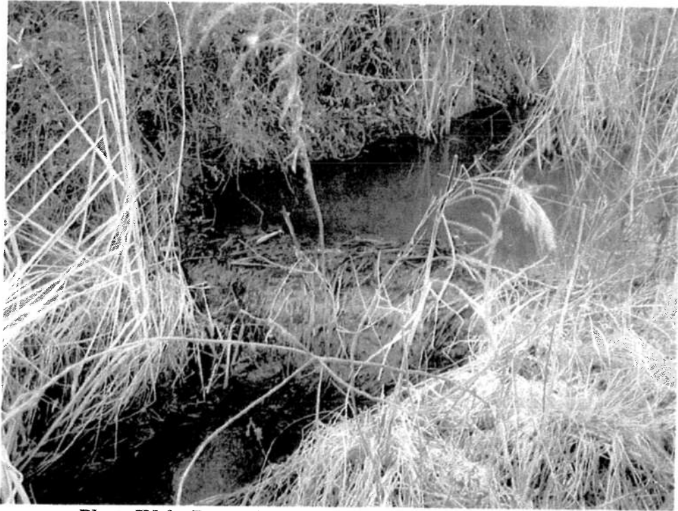
Photo IN-3: Beaver Dam in Drain Along Toe of North Dike
