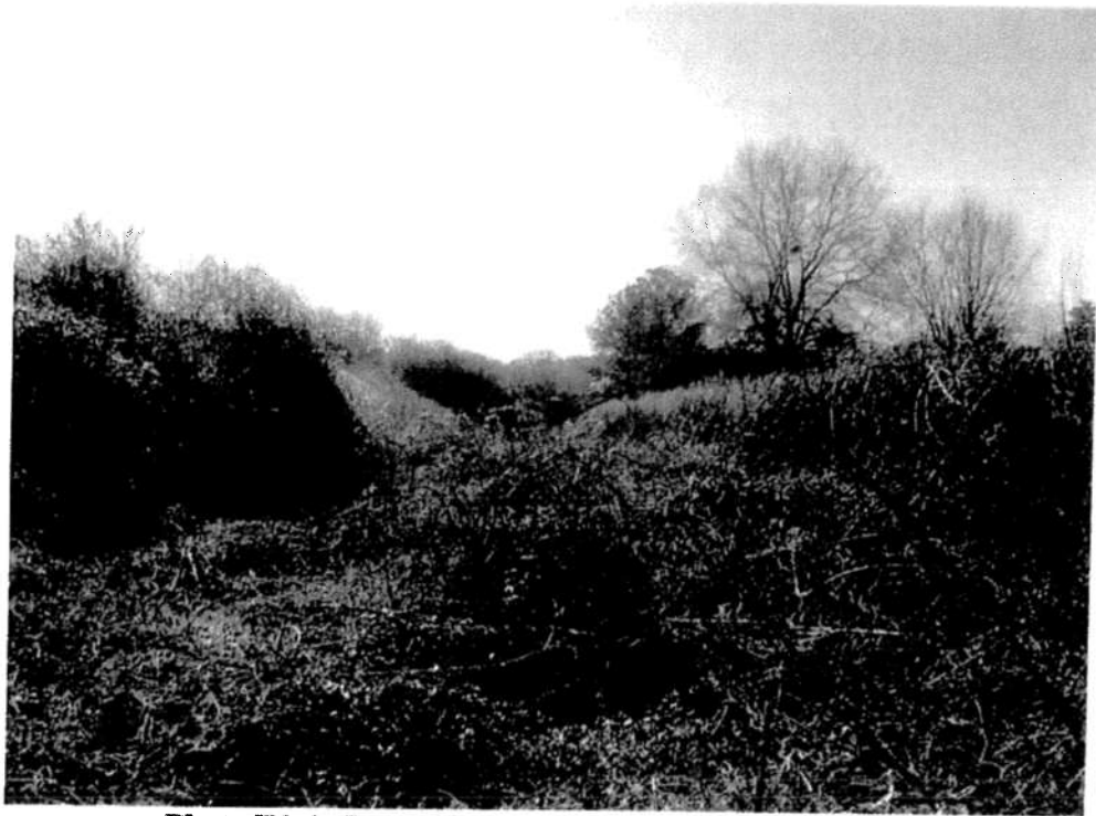
Photo IN-6: Dense Vegetation Along Toe of West Dike
