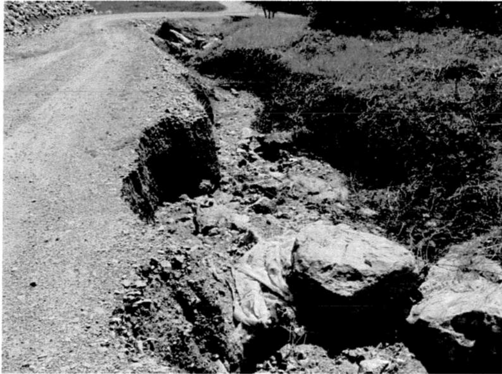
Photo 11 – Erosion of Road to Discharge Outlet Structure
