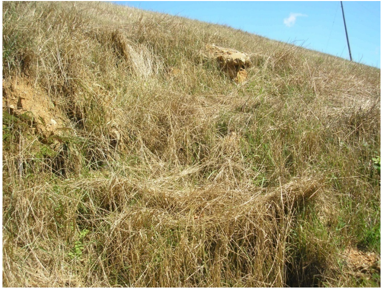
Photograph 15: Slump Top Slope East Dike, 6/23/2010
