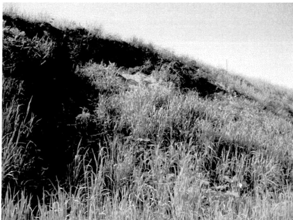
Photo 4 – Shallow Slide on Face of North Dike Requiring Repair
