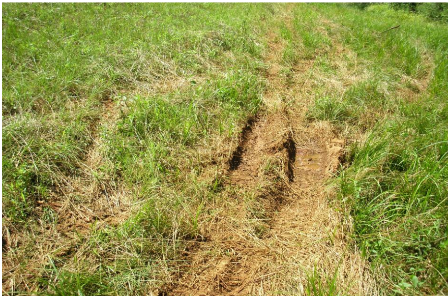
Figure 5.2.3-7 Photo Showing Small Wet Area West Dike Downstream Toe
