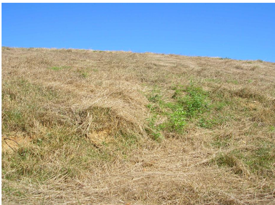
Figure 5.2.3-2 Photo Showing Small Area Mid-Slope Sloughing on East Dike Downstream Slope
