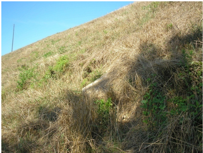
Photograph 12: Erosion Seep - Mid-slope East Dike, 6/23/2010
