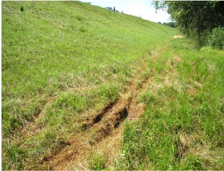
Photograph 25: West Dike Soft Wet Area at Toe, 6/23/2010
