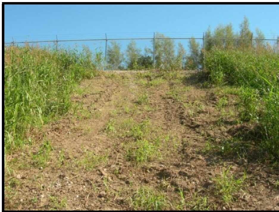
Figure 13: Ash pond exterior embankment erosion.
