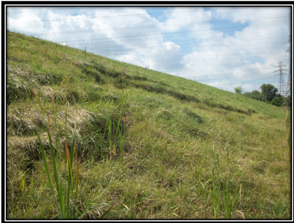
Photo 38 – Scarp on Western Pond 1 Downstream Slope
