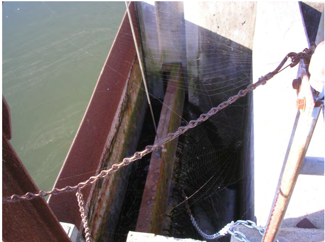
Figure 5.5.1-2: Ash Settling Pond Primary Spillway Structure Inflow Gate Control Lift
