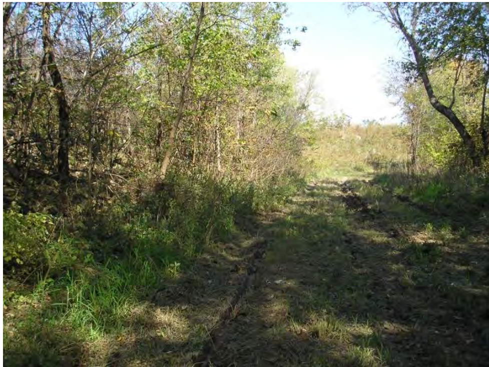
Figure 5.2.3-5: Wet Area at Ash Settling Pond South Dike Down Gradient Toe
