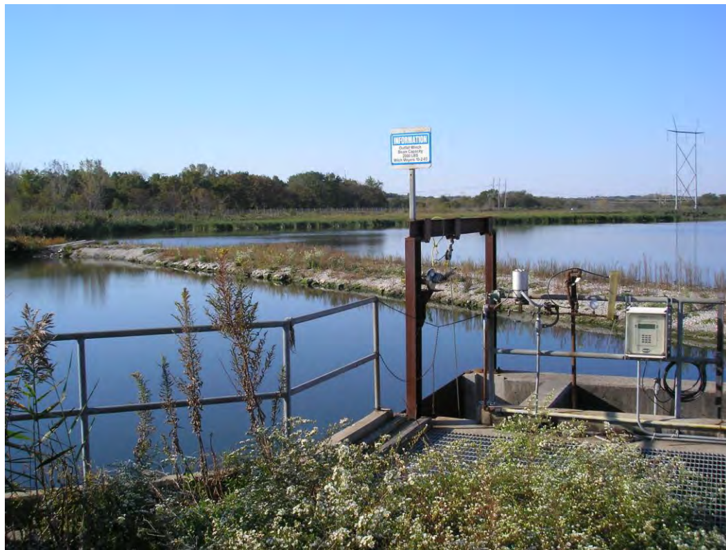
Figure 4.2.1-1: Ash Settling Primary Spillway Structure and Low Dike for Polishing Basin
