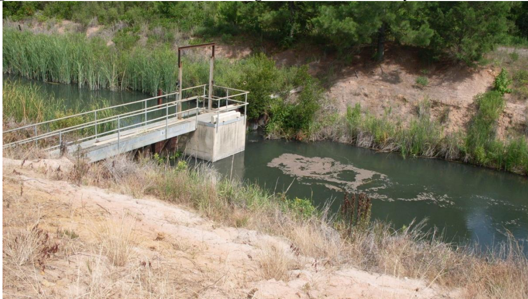
Figure 5-5: 48" Outlet Box and Discharge Channel of Primary Ash Pond
