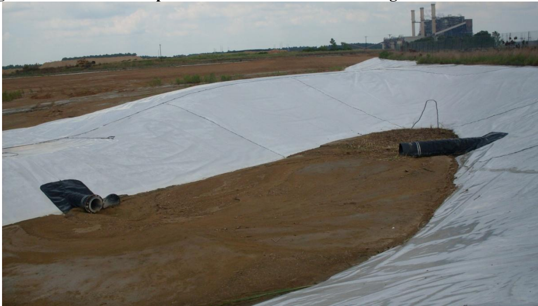
Figure 5-9: 30" Outlet Pipe from Active Bottom Ash Storage Pond
