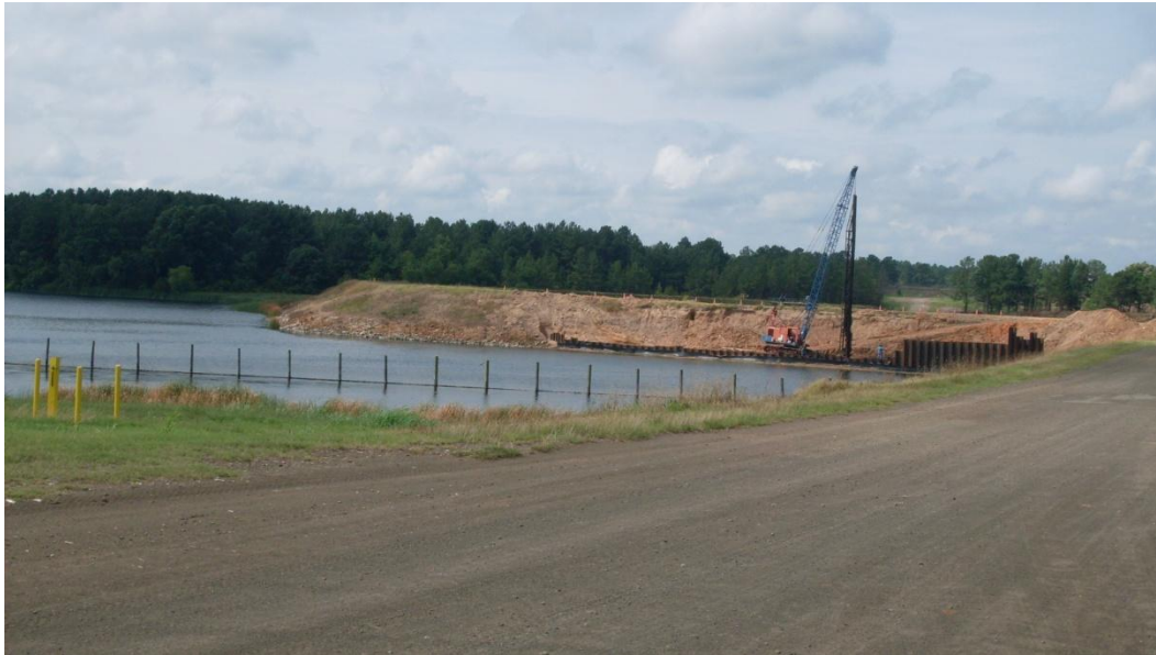
Figure 5-1: Crest around East End of Primary Ash Pond with gravel access road way
