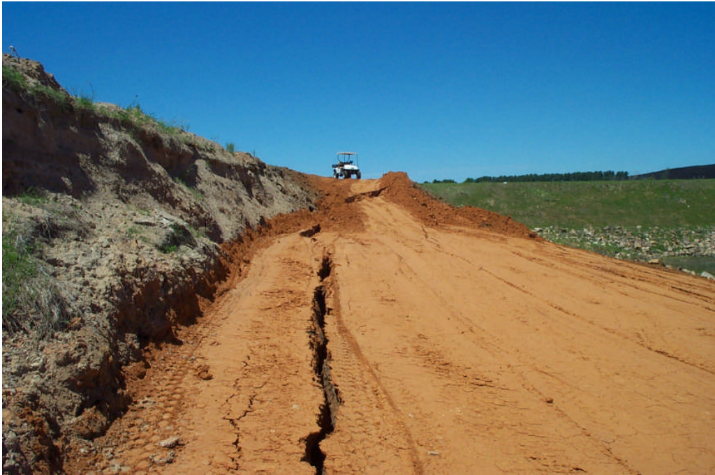
Photo 3 Slipping of Repair Surface
