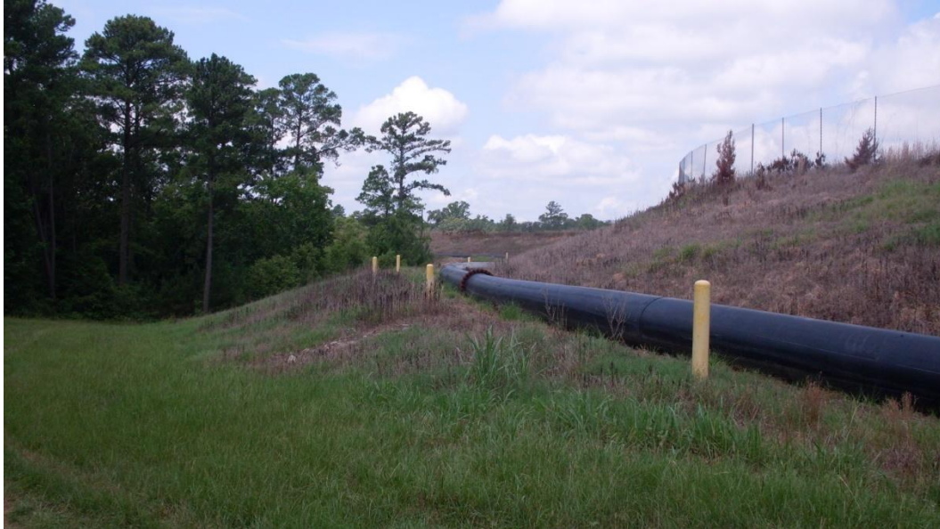
Figure 5-15: 30” HDPE Outlet Pipe Recirculating Supernatant from Active Bottom Ash Storage Pond to Primary Ash Pond
