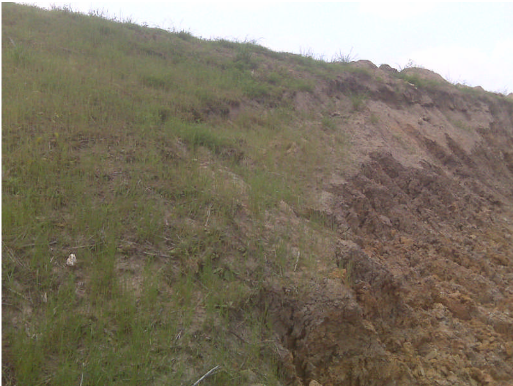
Photo 4 - Top of Failure Plane
