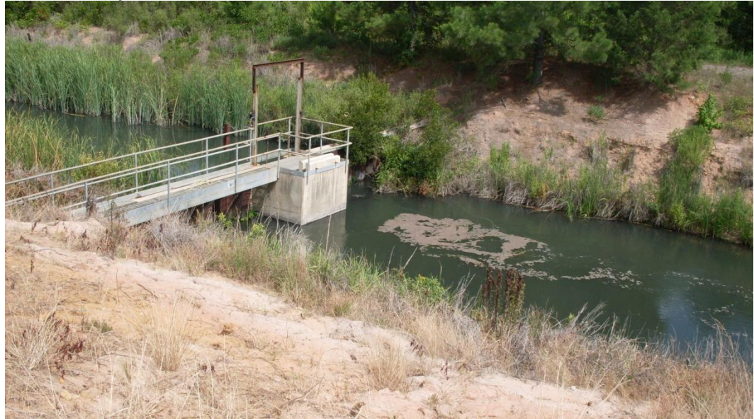
Figure 2-1: Primary Ash Pond Outlet
