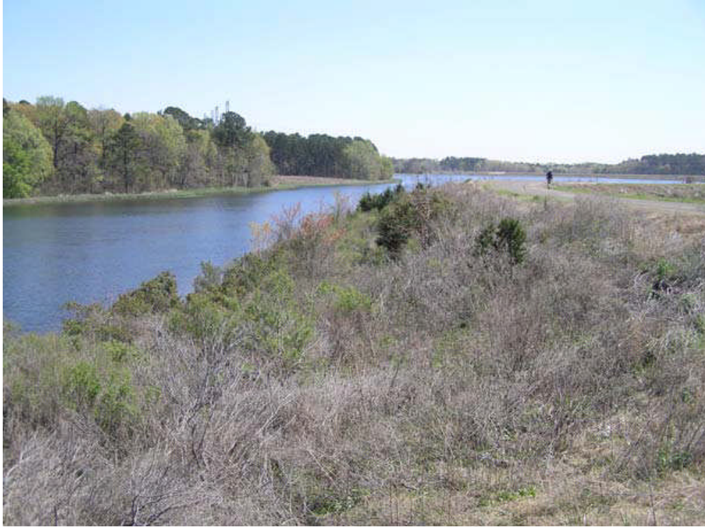
Photo 1 Original Embankment Before Slough
