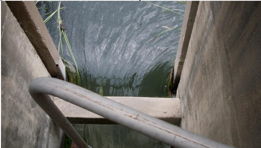
Figure 5-10: Effluent Outlet from Secondary Ash Pond
