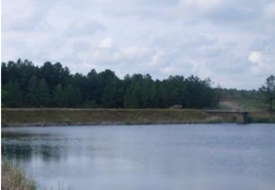
Figure 5-9: 48" Outlet Box in the Secondary Ash Pond
