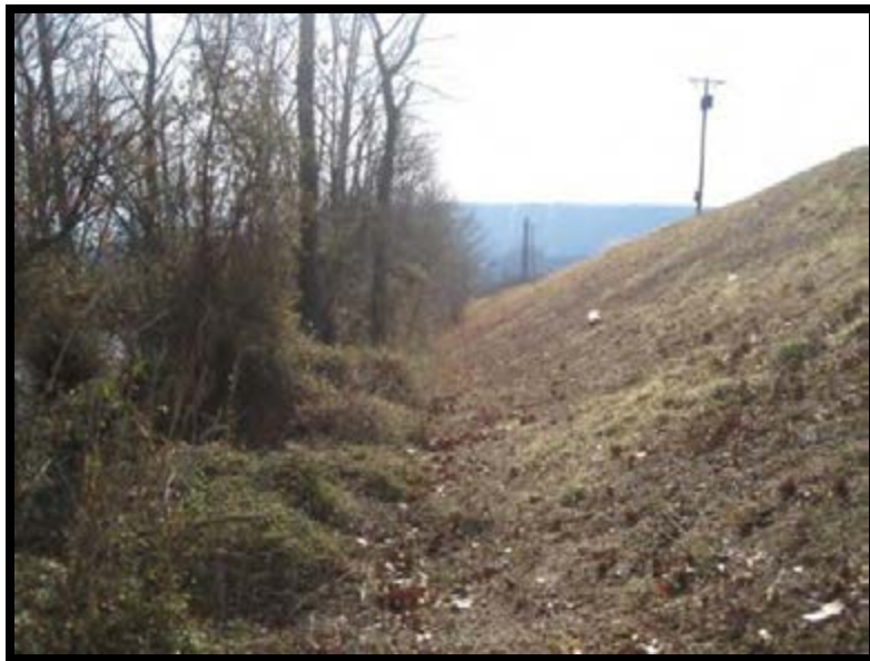
Figure 5.2.3-1: Downstream slope, Southeast. Note woody vegetation and trees growing at toe of the embankment.
