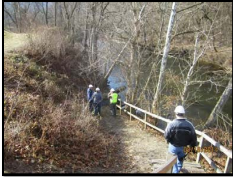
Figure 5.3.3-2: Downstream slope, East. East River to the right. Note woody vegetation and trees growing on dike.
