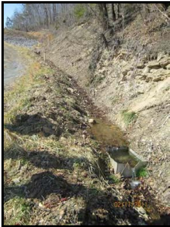
Figure 5.2.4-1: North abutment ditch. Note upstream riprap and v-notch weir used to monitor seepage.
