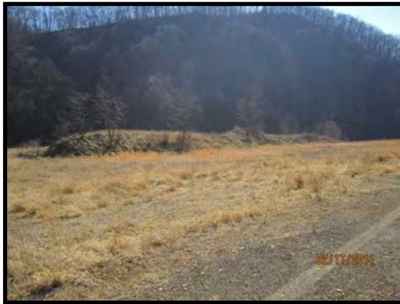
Figure 5.3.3-1: Remaining portion of upper dike, Southeast. Note tree growth on downstream slope.
