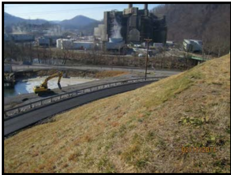
Figure 5.2.3-2: Downstream slope along paved access road, Southwest. Note reclaim beyond the toe of the perimeter dike.
