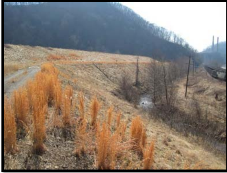
Figure 5.3.3-2: Downstream slope of lower dike, Southeast. Note significant tree growth along Dumps Creeks.
