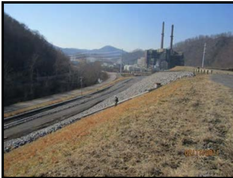
Figure 5.2.3-3: Downstream slope, Southwest. The embankment runs parallel to Route 616. Note transit pipes along edge of riprap. Transit pipes carry offsite runoff through the ponds splitter dike and out to Dumps Creek.
