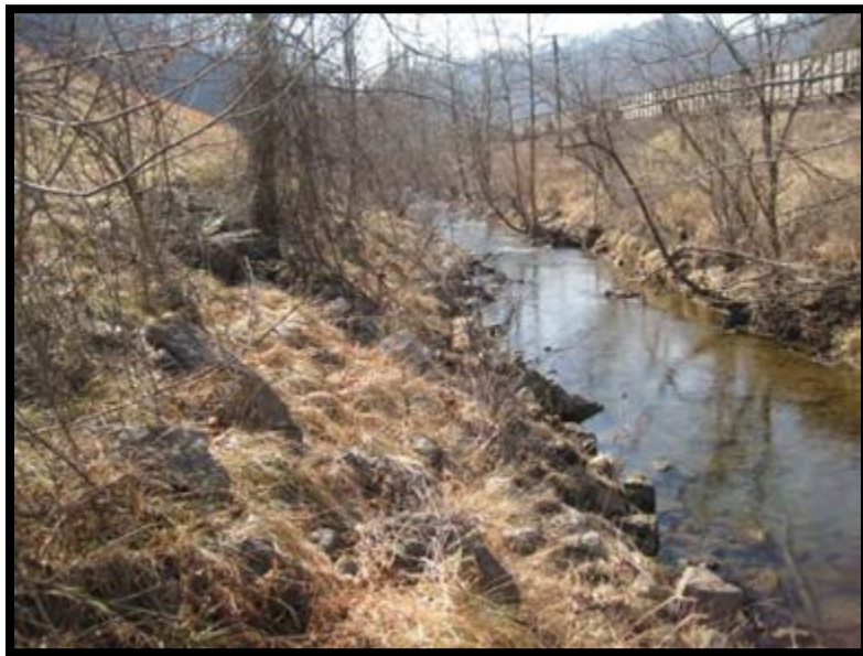
Figure 5.3.3-3: Downstream toe of lower dike. Note significant tree growth and rip-rap adjacent Dumps Creek.
