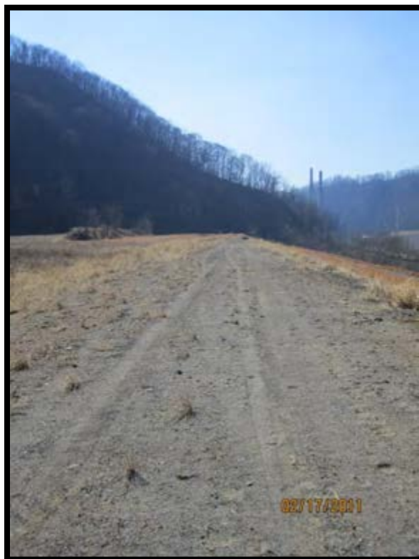
Figure 5.3.1-2: Middle dike crest, South. Note removed portions of upper dike and re-grading near crest of the middle dike.
