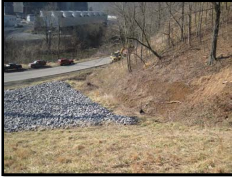
Figure 5.2.4-2: South abutment ditch. Note downstream slope rip-rap used for seepage control and abutment ditch used to convey hillside drainage.
