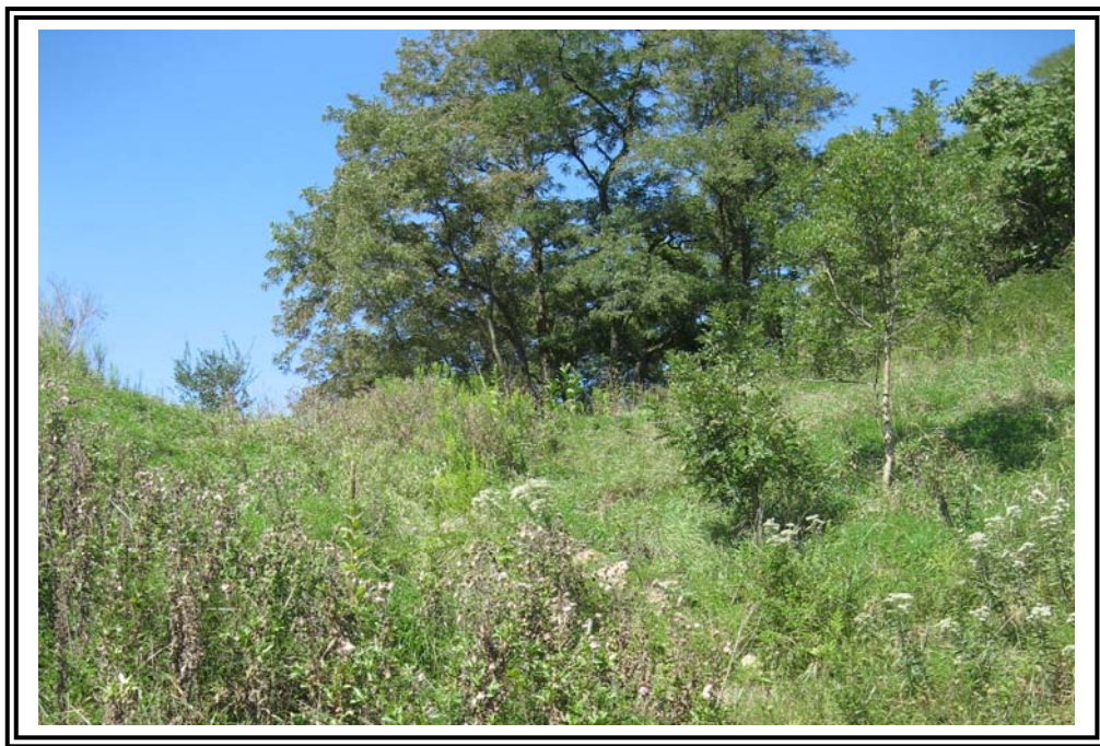
Left (north) abutment rock groin; heavily vegetated.
