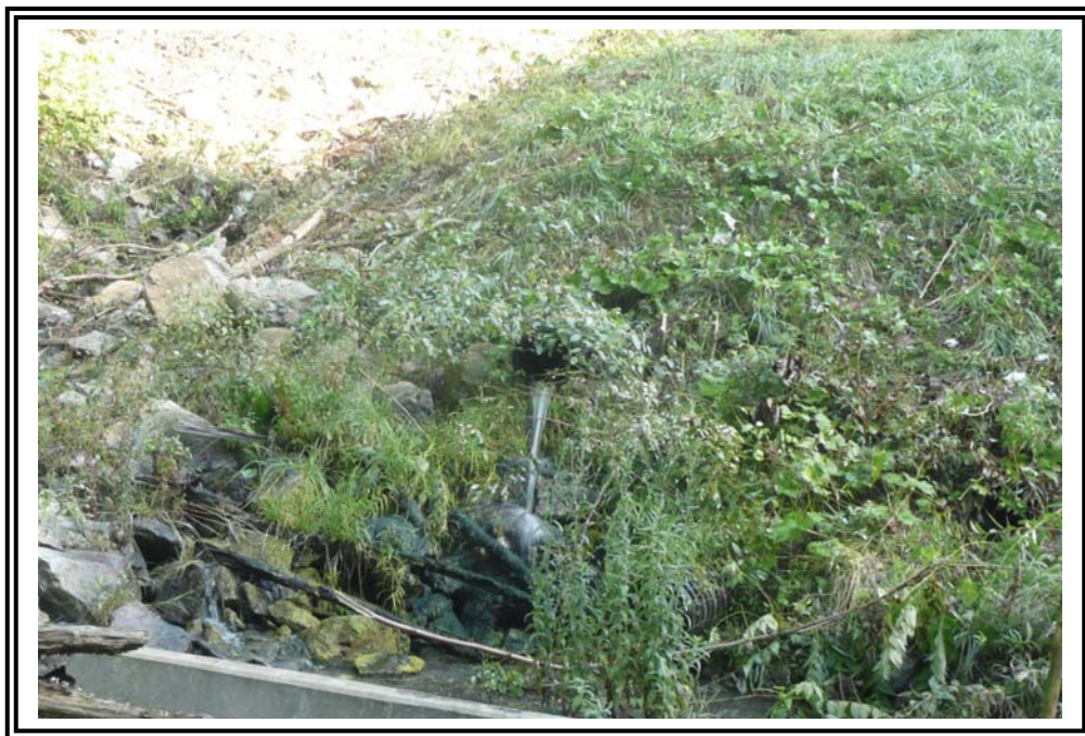
Closer view of seepage discharge.
